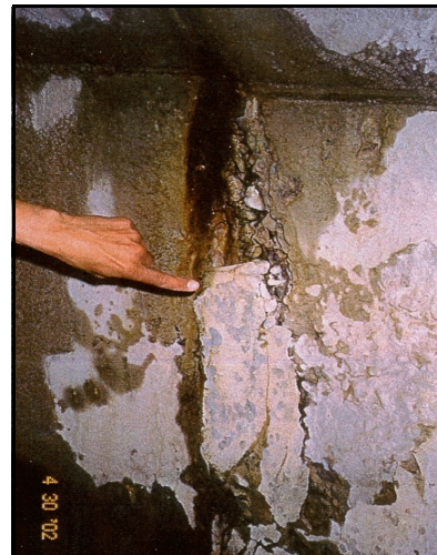
Figure 193. —Determine the cause of the damage to determine the proper repair method.
