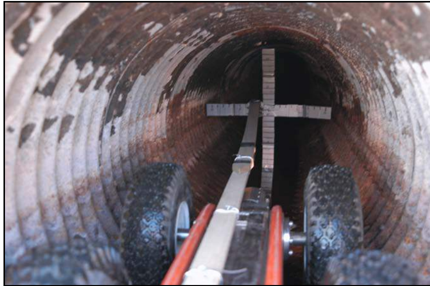
Figure 160. —Crossbar template attached to a CCTV camera-crawler to check for irregularities in the CMP conduit.
