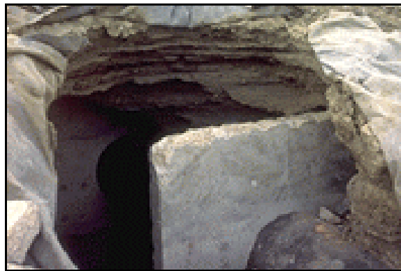
Figure B-2. —A view of upstream end of outlet conduit following failure. Note formation of caverns immediately adjacent to seepage cutoff collars. These caverns extend to the downstream embankment toe.
