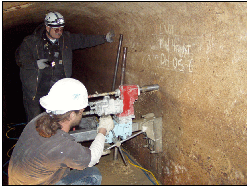
Figure 143. —A core hole is being drilled to reveal voids behind the concrete in this conduit.
