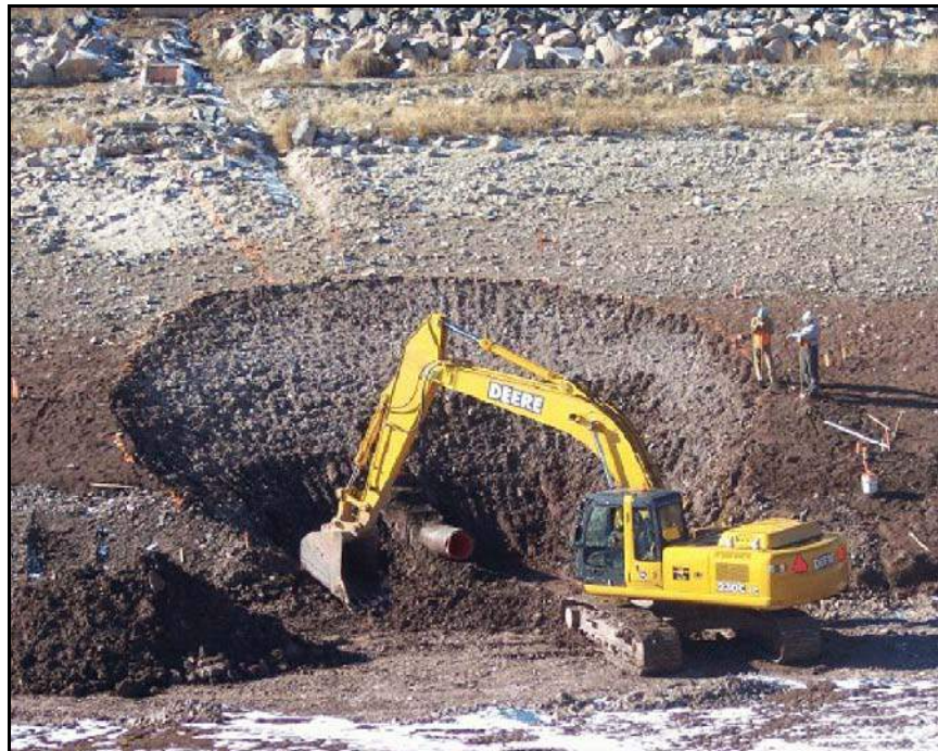
Figure 170. —The intake structure has been removed as part of a conduit renovation.
