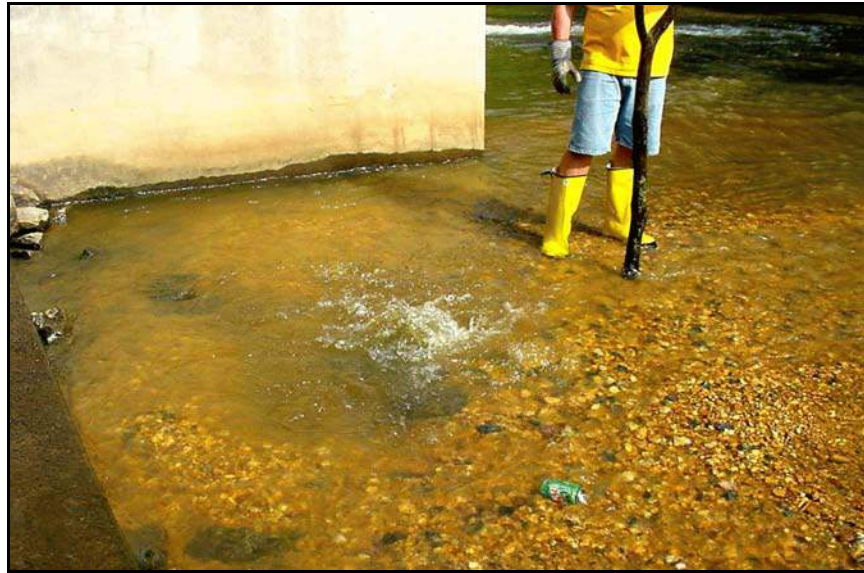
Figure B-28. —Seepage flow at the downstream end of the spillway appeared to be boiling. Attempts to create a sandbag weir around the boil to reduce leakage under the spillway were unsuccessful.
