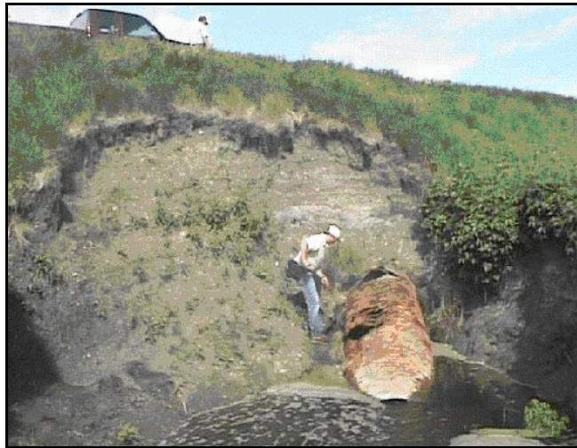
Figure 113. —An outlet works conduit that has experienced corrosion and failure.
