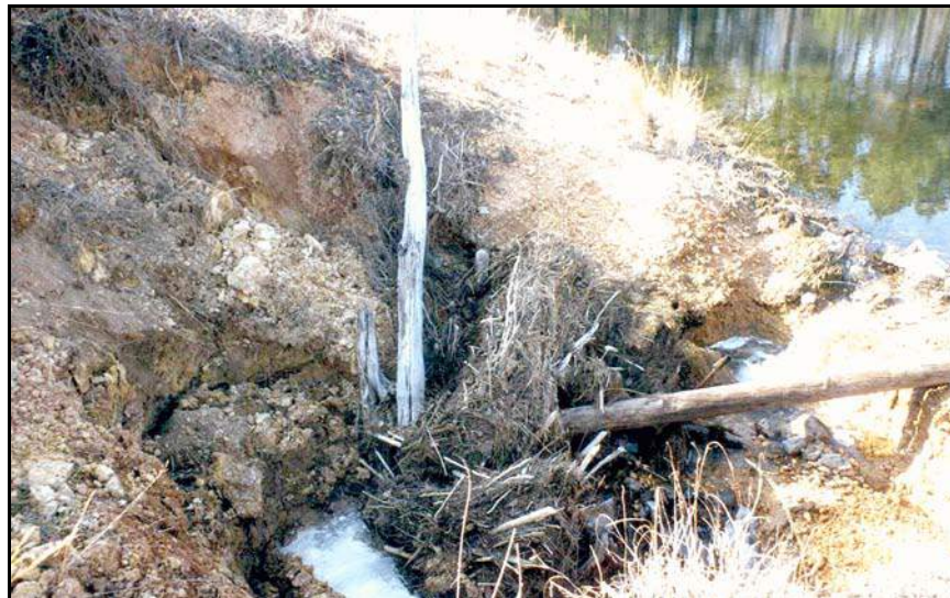
Figure 154. —Care must be taken to ensure that debris does not clog spillway after removal of the riser.
