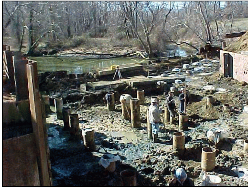
Figure B-24. —Because of soft foundation soils, numerous 60-foot long pipe piles were installed in winter 2001 to support a new reinforced cast-in-place concrete spillway structure.
