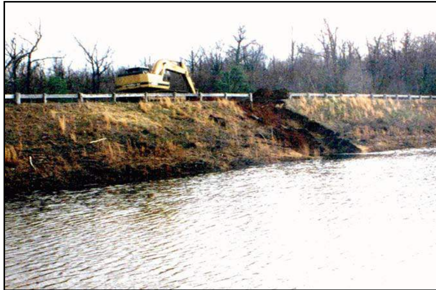
Figure 157. —A controlled breach of an embankment dam begins after the 45-year old CMP spillway conduit collapsed and the lake level began to rise.
