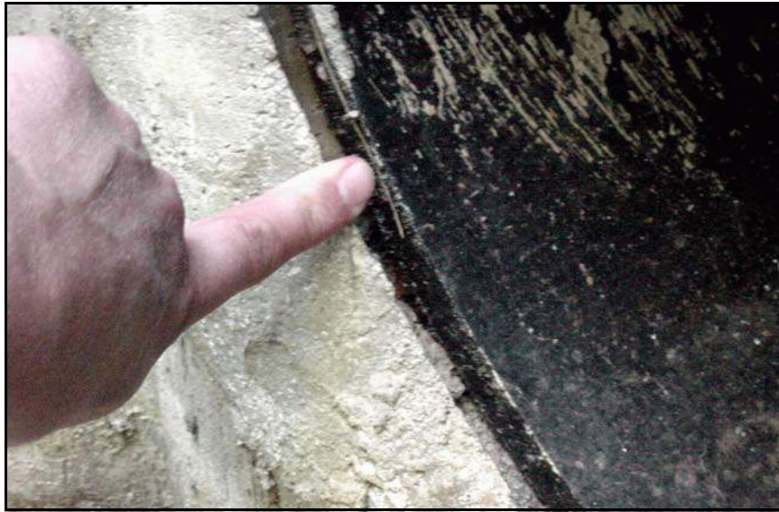
Figure 175. —This gap shows that the designer did not adequately consider the potential for thermal expansion/contraction during installation of this HDPE slipliner. To avoid this problem, the HDPE slipliner should have been designed to extend beyond the end of the existing conduit.
