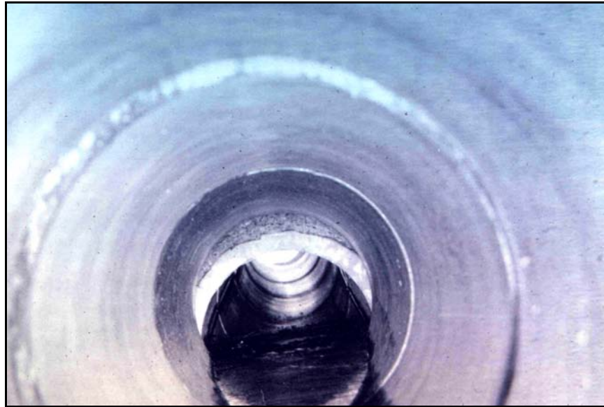
Figure 117. —This conduit was severely damaged after the foundation settled more than 2 feet.
