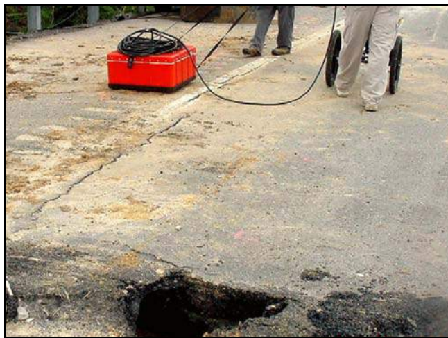
Figure B-31. —Ground penetrating radar identified the location of voids along the CMP.
