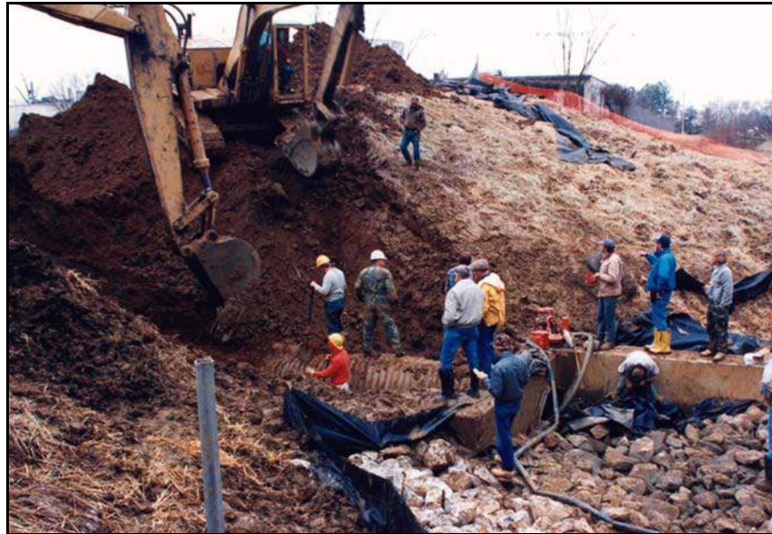
Figure B-7. —The spillway conduit and portions of the embankment soils were carefully removed and documented during a forensic investigation about 2 weeks after the failure.
