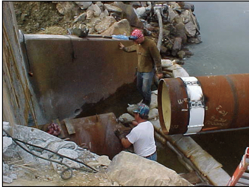
Figure 180. —The Lake Linganore Dam outlet works consists of a 48-in diameter RCP conduit with a sluice gate located at the downstream end, which places the conduit under full reservoir head at all times. Concern about the integrity of the RCP joints led to installation of a steel slipliner when the inoperable sluice gate was replaced.
