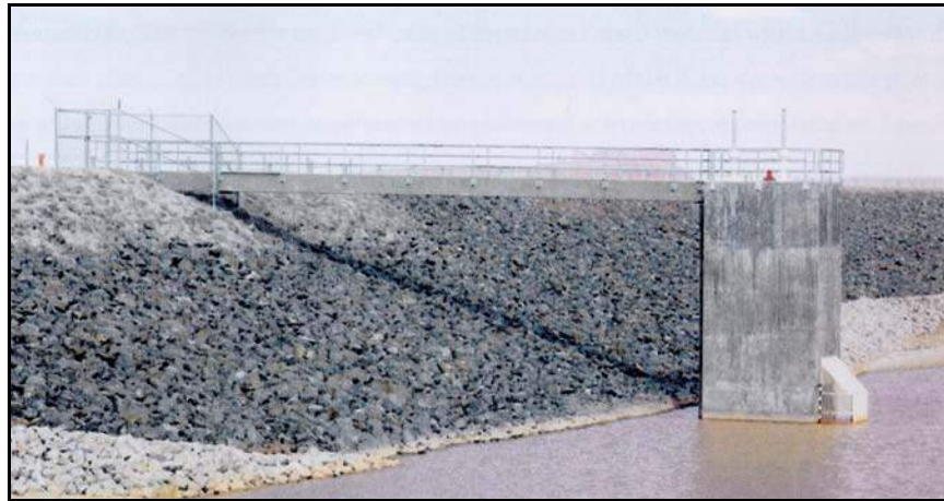
Figure 42. —Typical outlet works intake structure.
