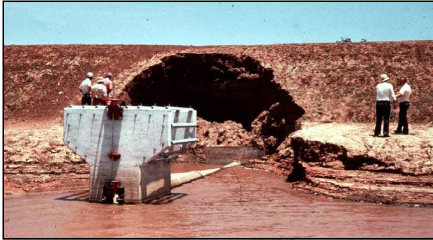
Figure 5. —Embankment dam failure caused by internal erosion of earthfill near the conduit. Flow was not directly along the contact between earthfill and conduit, but in the earthfill away from conduit. Hydraulic fracture in highly dispersive clay embankment soils caused the failure. The embankment design included antiseep collars, but not a filter diaphragm.
