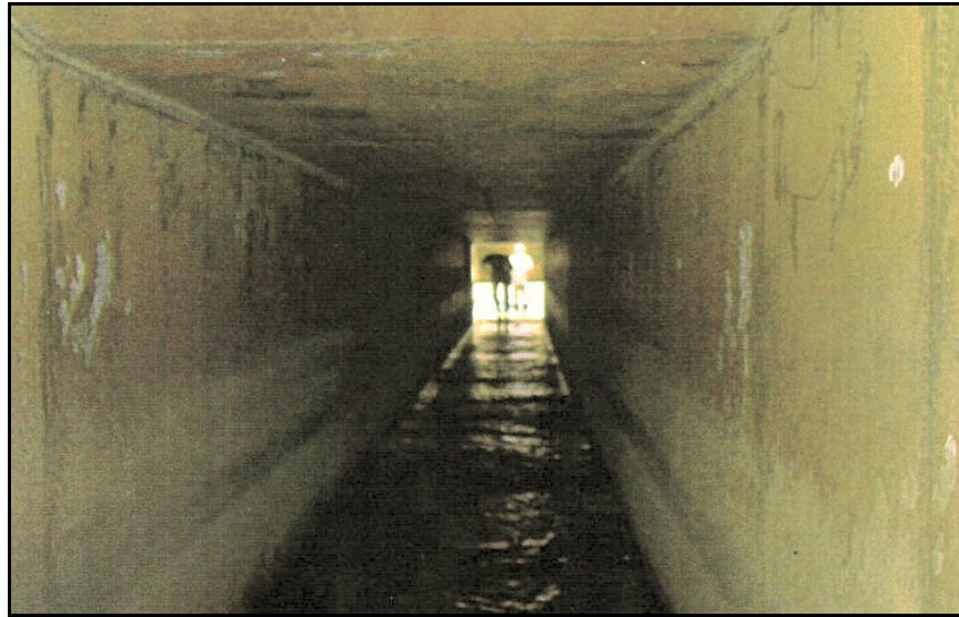
Figure 59. —A box shape is not commonly used for conduits. The designer needs to carefully consider the advantages and disadvantages of this shape.
