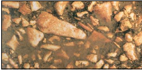
Figure 105. —Abrasion/erosion damage to concrete from flowing water containing sand and silt.
