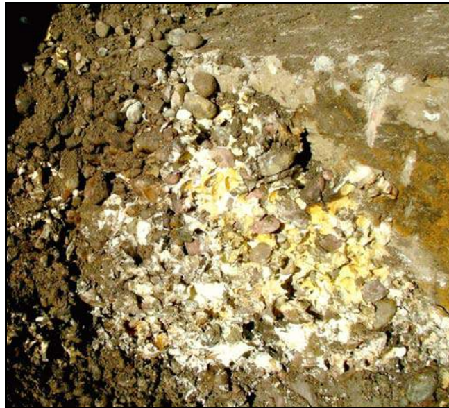
Figure 136. —Close coordination between the forensic team and contractor allowed for careful study of how polyurethane grout injected into the deteriorated joints of a conduit flows through surrounding backfill. In this case, the forensic investigation showed the injection of grout was relatively successful in sealing the joints of the conduit.
