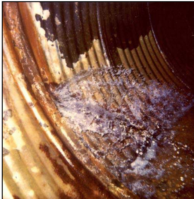
Figure 98. —Leakage from an unauthorized “field joint” constructed by the contractor about 5 feet downstream from the spillway riser structure. An inspection revealed that nearly all of the joints were exhibiting severe leakage and loss of embankment material.
