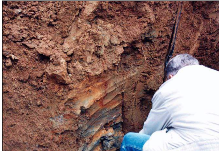
Figure B-10. —The presence of undisturbed foundation soils confirmed that the conduit was placed in a trench with nearly vertical sides, making it difficult to obtain good compaction of the fill soils under and along the CMP and around the antiseep collars.
