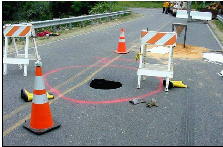
Figure B-26. —Less than 2 years later, an engineer inspecting the bridge over the spillway reported that seepage flow was visible from under the downstream end of the spillway. The seepage flow was clear, and no migration of soils was evident. A few months later, the roadway on the dam crest collapsed, and large quantities of sediment were observed in the pool below the dam.
