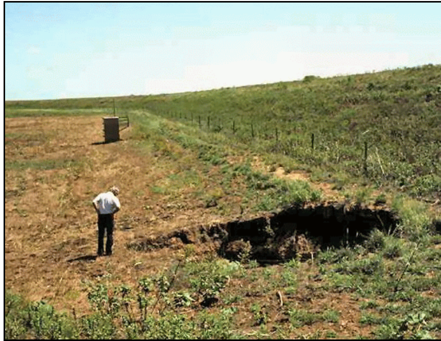
Figure 119. —Sinkhole in the crest of an embankment dam.
