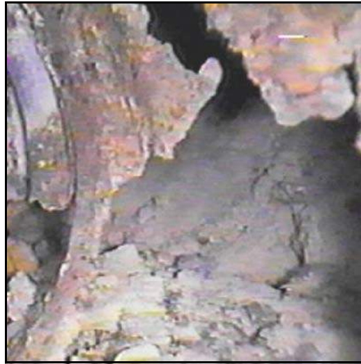
Figure 109. —Corrosion has completely destroyed this CMP spillway conduit. Backfill materials that surrounded the conduit have been eroded by flow within the conduit.
