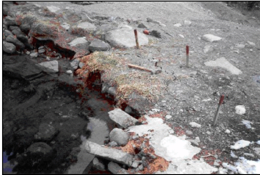
Figure B-16. —Cracking at the embankment dam crest above the sinkhole on the upstream slope of the embankment dam. Note the simple staking of the area to monitor movement of the crack.
