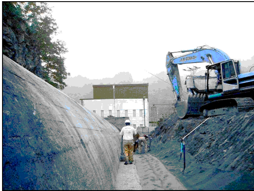
Figure B-79.—Filter material being placed in thin lifts and compacted with hand-operated vibratory compaction equipment.
