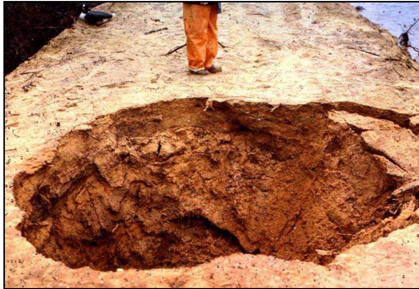
Figure 147. —Sinkhole over a spillway conduit.
