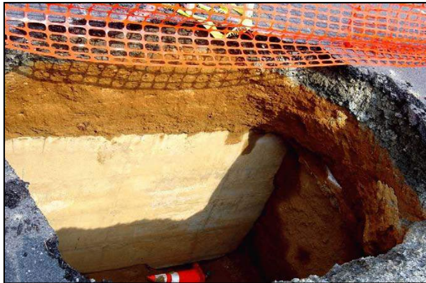
Figure B-27. —The road was closed immediately, and lake level was lowered. However, the sinkhole rapidly enlarged.
