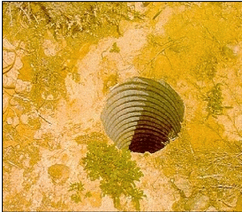
Figure 44. —No intake structure exists for this outlet works. This conduit is prone to plugging with trash and debris.
