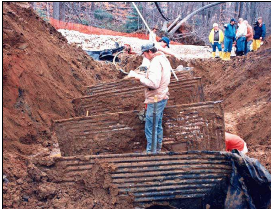
Figure B-11. —Seepage along the sides of the CMP resulted in loss of soil support, causing conduit and joint deformation.
