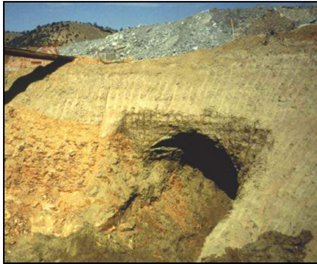
Figure 149. —Incipient sinkhole in an embankment dam. Eventually, the continued removal of the soil at the bottom of the cavern would have caused the roof to migrate to the surface of the embankment dam.
