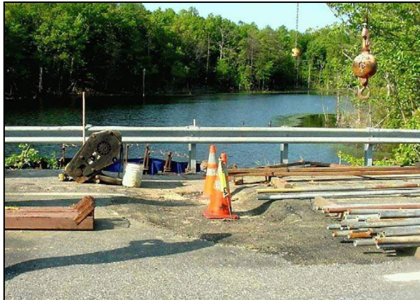
Figure B-29. —A sinkhole, which appeared in a heavily traveled roadway above a 20-year old CMP spillway, was filled with asphalt. Part of the roadway was closed when the asphalt patch subsided a few hours later.
