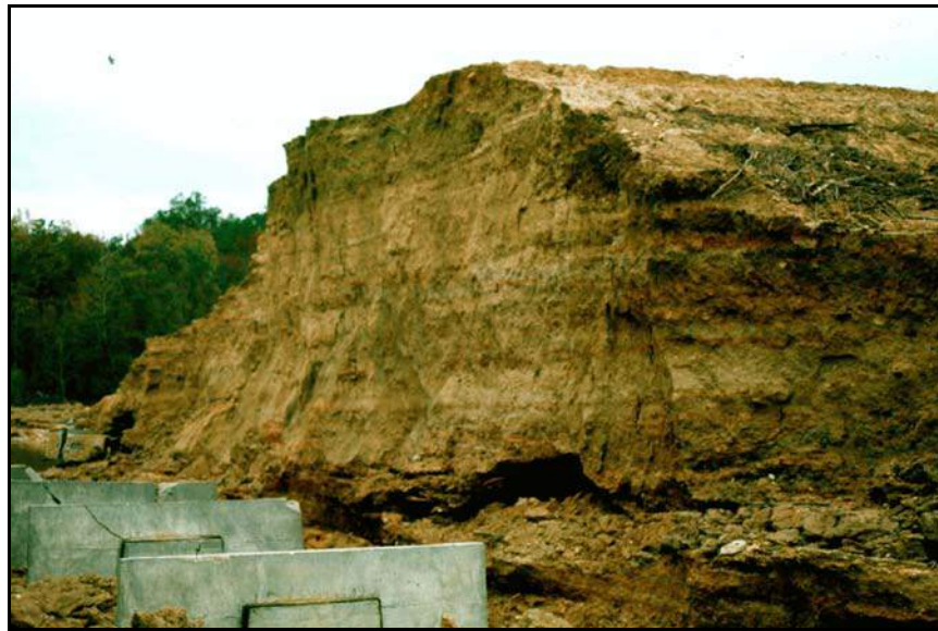
Figure 82. —The failure of this embankment dam located in South Carolina was attributed to hydraulic fracture. The eroded seam located to the right of the conduit may have been the hydraulic fracture that formed and allowed internal erosion and failure of the embankment dam. The embankment was composed of dispersive clays.
