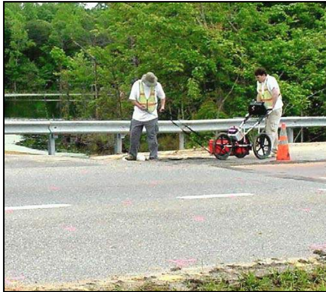
Figure B-30. —Ground penetrating radar investigations were performed from the embankment dam crest.
