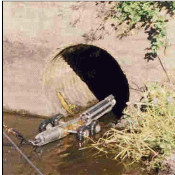
Figure 128. —A CCTV inspection camera-crawler entering the downstream discharge portal of an outlet works conduit.
