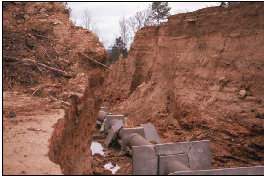
Figure 17. —Failure of an embankment dam following first filling. The failure was attributed to internal erosion because the time required for seepage to develop through the compacted embankment and cause failure was very short. Also, the soils are not the type ordinarily considered susceptible to backward erosion piping. Antiseep collars were not effective in preventing the failure.
