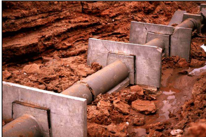
Figure 102. —Conduit with intact antiseepage collars. The collars would have interrupted flow along conduit. Internal erosion or backward piping erosion likely occurred through hydraulic fractures in surrounding earthfill, resulting in failure of this embankment dam.
