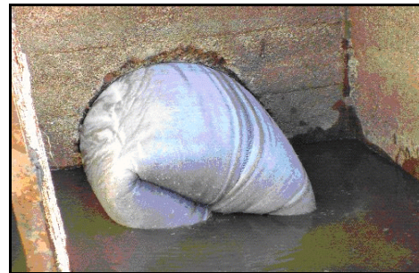
Figure 184. —The hydrostatic inversion method is being used for CIPP liner installation into an existing conduit.
