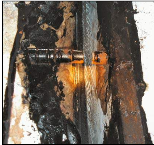
Figure 63. —Longitudinal reinforcement across a conduit joint experienced tensile failure caused by lateral spreading of the embankment dam.
