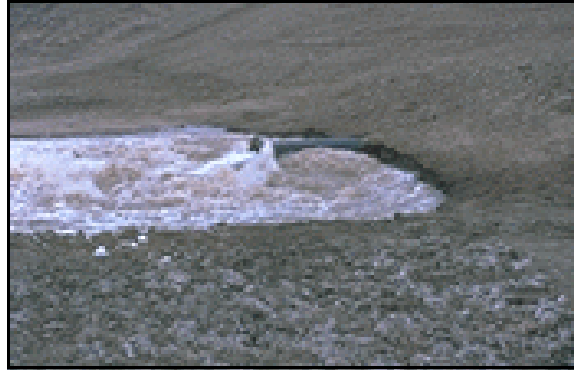
Figure B-1. —Outflow of water at downstream end of outlet conduit during failure. Note flow from conduit itself and from the area adjacent to the conduit.
