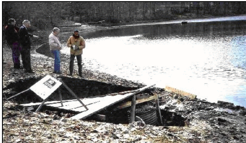
Figure B-67. —When the 35-year old corrugated metal pipe riser collapsed, a large portion of the low hazard embankment dam was washed away. This left a void about 30 feet in diameter and 10 feet deep around the original riser.
