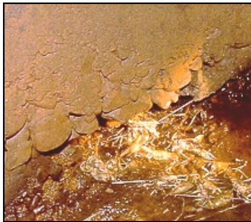
Figure 115. —A rock pocket at the bottom of a conduit side wall.
