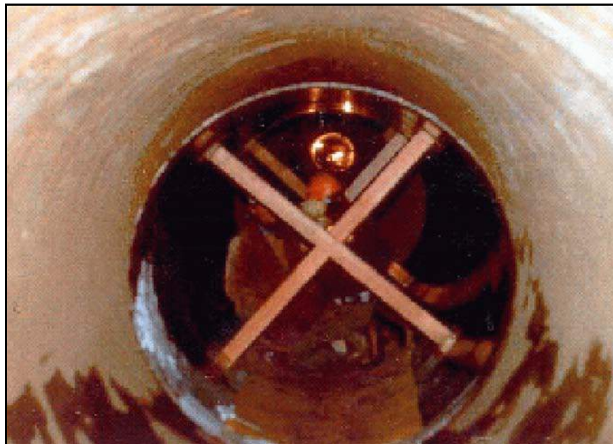
Figure B-34. —Installing the steel pipe slipliner within the existing outlet works conduit.
