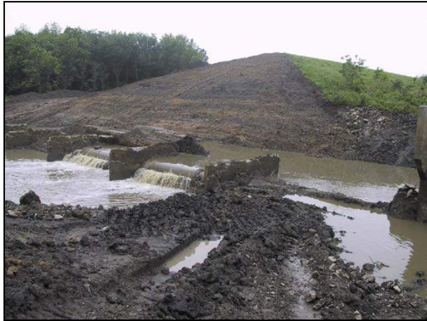
Figure 188. —During the removal of this outlet works conduit a flood occurred. No stream diversion or cofferdam was used at this site.
