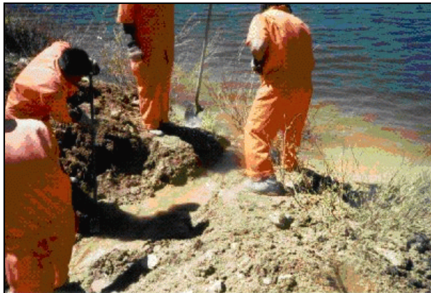
Figure B-39. —Completion of the initialization of the breach in the embankment dam.
