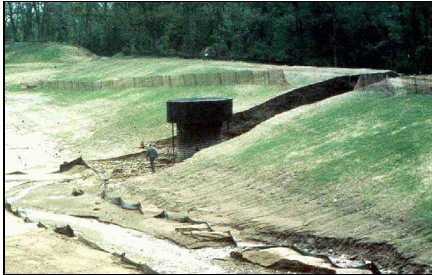
Figure B-50. —Loveton Farms Dam failure as viewed from upstream. Note that the walls of the failure area are nearly vertical. The construction records indicate that a large portion of the embankment dam was placed prior to installation of the CMP.
