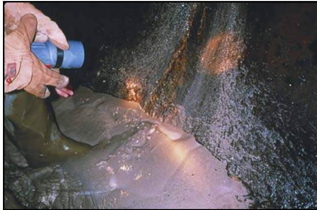
Figure 97. —Soil particles being carried into an outlet works conduit through a joint.
