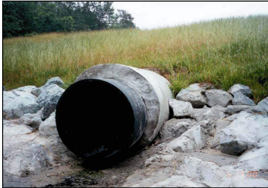
Figure 176. —Completed HDPE slipliner in existing CMP spillway conduit. Photo courtesy of Maryland Dam Safety Division.
