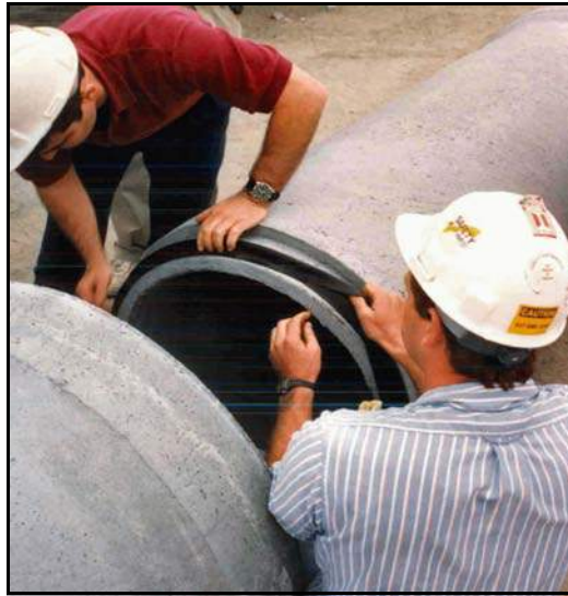
Figure 79. —A rubber gasket is installed at the spigot end of the precast concrete pipe.
