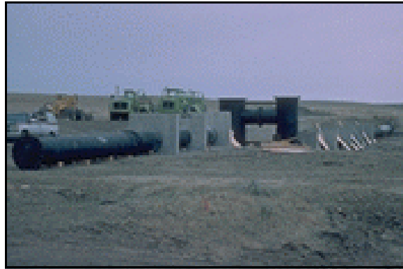
Figure B-3. —Initial construction of embankment dam and outlet conduit (upstream is to left). Note presence of antiseep collars surrounding conduit.
