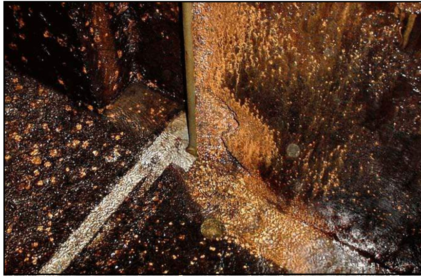
Figure 108. —Cavitation damage to the cast-iron lining of a conduit immediately downstream of a slide gate, caused by high velocity flow.
