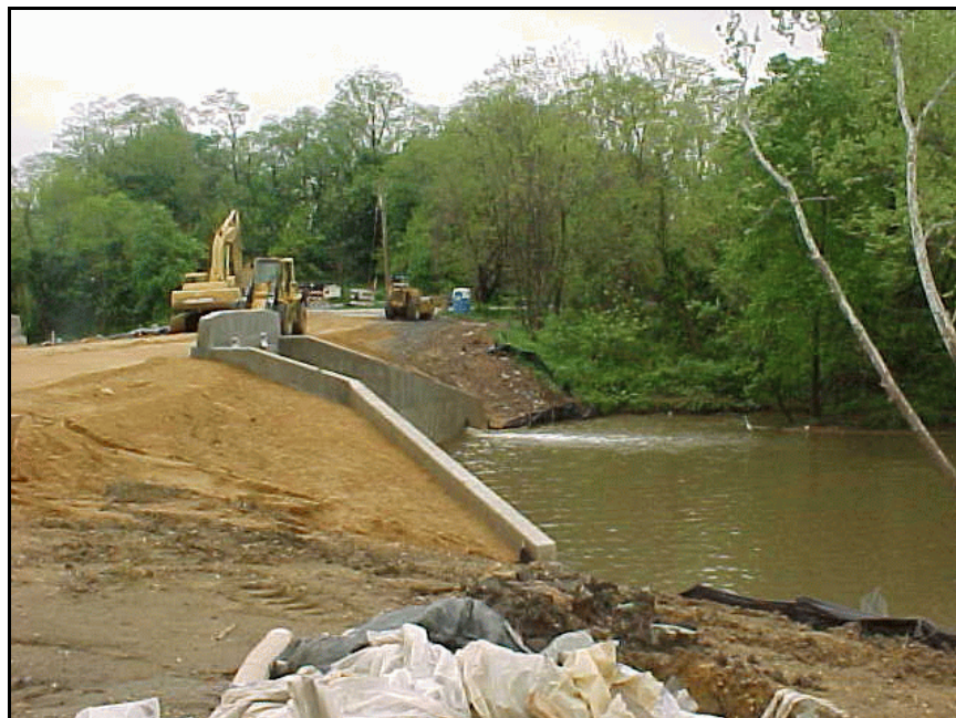
Figure B-25. —This the downstream end of the spillway at the end of construction in 2002.
