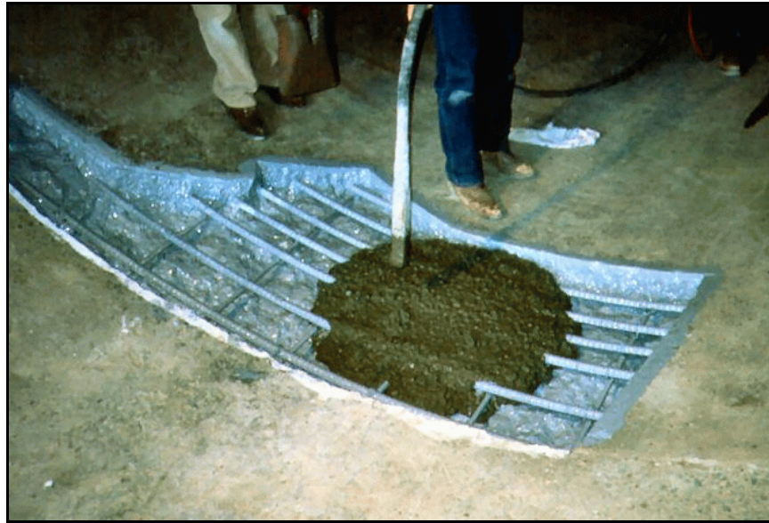
Figure 195. —A repair being made using epoxy-bonded replacement concrete. The use of epoxy resin ensures a strong, durable bond between the old concrete and the replacement concrete.
