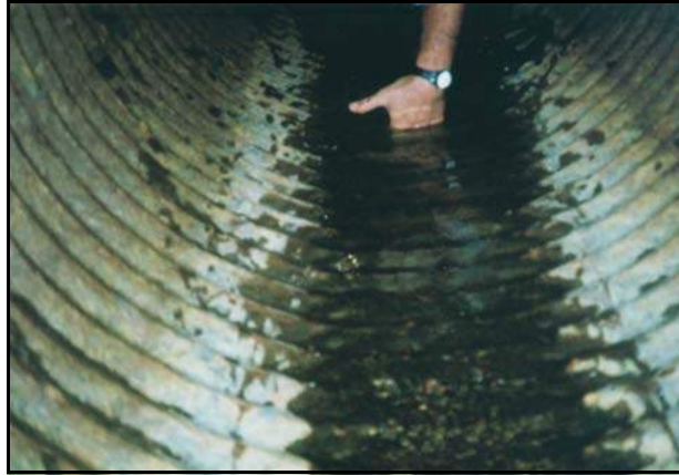
Figure 111. —CMP corrosion on the invert of an outlet works conduit.
