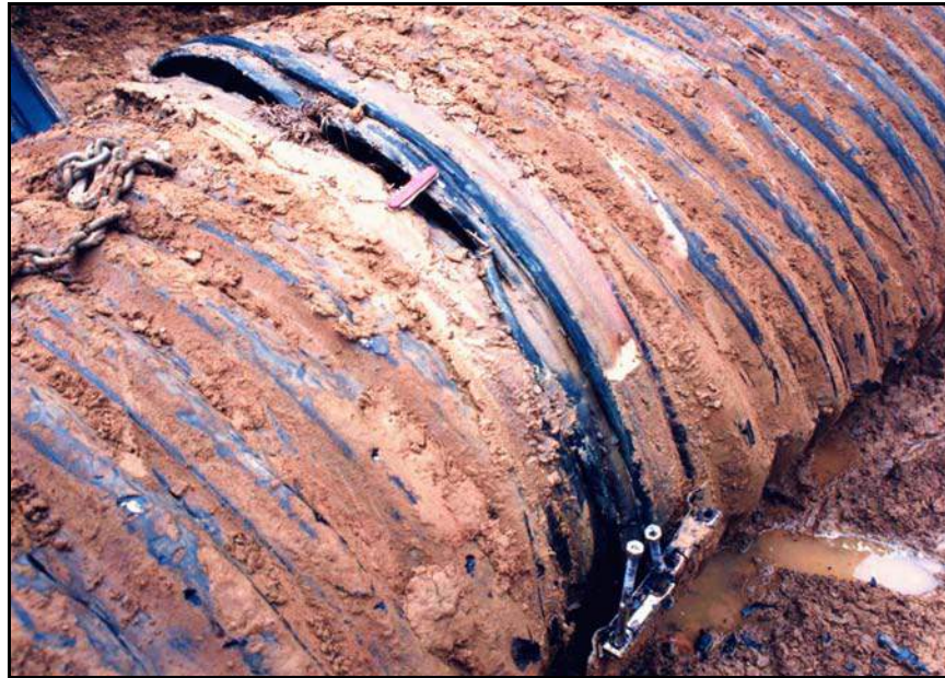
Figure B-9. —When the “hugger band” at the most downstream conduit joint was removed, the o-ring gasket was found to have been displaced. In addition, debris from the pool was found under the band, indicating that water may have flowed unrestricted along the outside of the conduit from the pool and into the joint.
