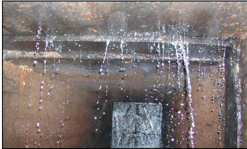
Figure 70. —Water seeping through a joint in an outlet works conduit. The joint has experienced differential settlement. This joint had no longitudinal reinforcement extending across the joint. The mortar joint filling has cracked and deteriorated.
