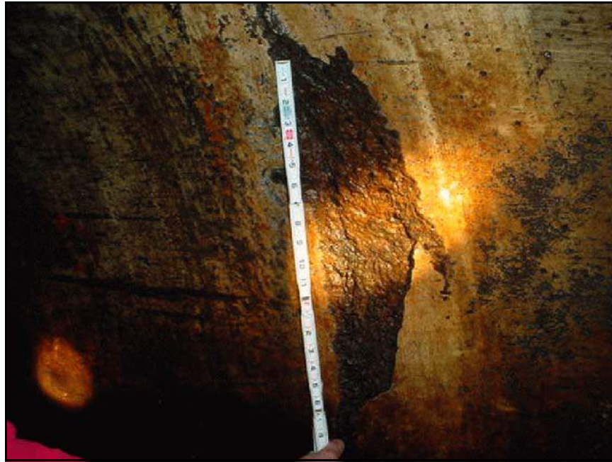
Figure B-20. —Large spall at the construction joint located at station 12+13.
