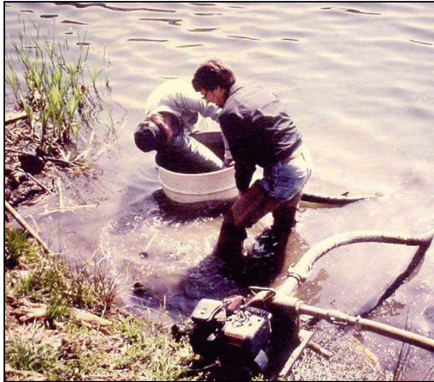
Figure 153. —The upper portion of a small metal pipe riser structure was removed with an acetylene torch. The riser was isolated from the pool by surrounding it with a large drum pressed into the soil. A pump was used to remove the water between the drum and the riser so that the work was completed in the dry.
