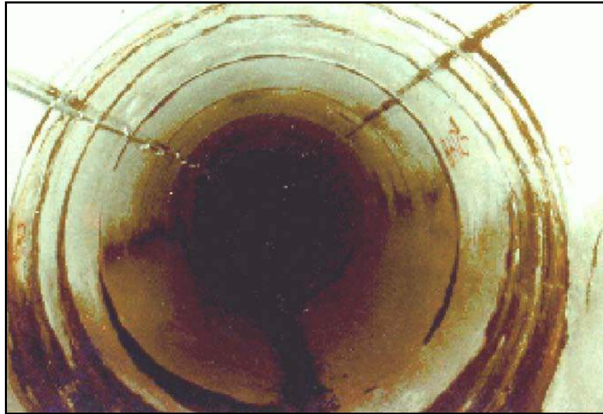
Figure B-66. —View of the interior of the outlet works after grouting.
