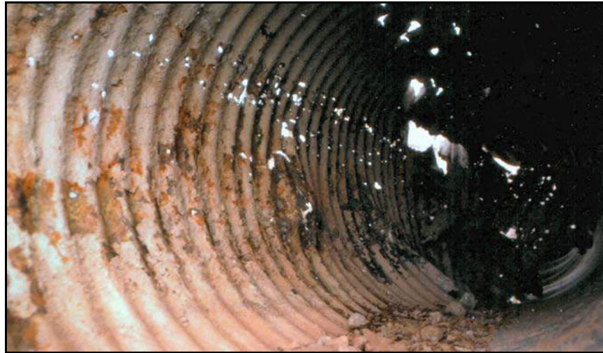
Figure 159. —The holes in this CMP conduit were clearly visible after removal. The conduit was considered to be so severely corroded that sliplining was not an option and it was removed and replaced. Photo courtesy of Maryland Dam Safety Division.
