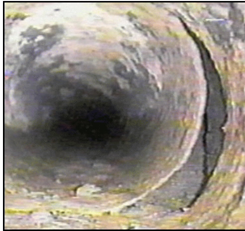
Figure 132. —A joint has separated in the steel pipe of this outlet works.
