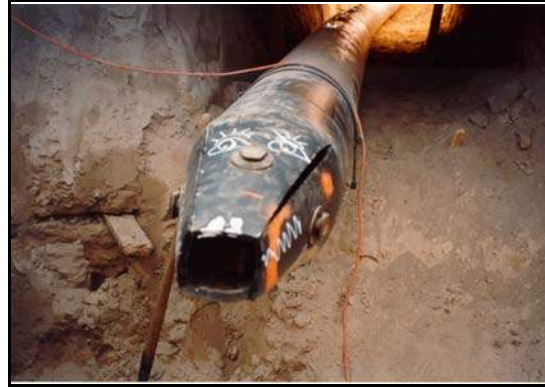
Figure B-76. —Upstream end of the HDPE slipliner modified to act as a pulling head.
