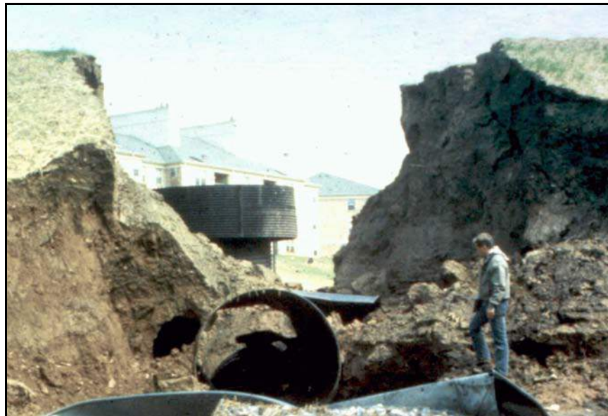
Figure B-51. —Loveton Farms Dam after failure as viewed from the downstream end of the 78-in diameter CMP spillway. Note that one of the antiseep collars, which were about 14 feet square, is visible in the breach.
