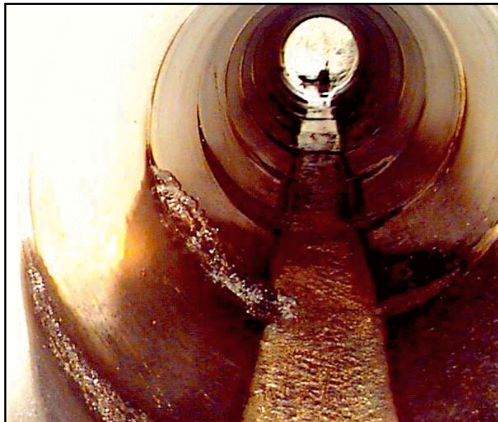
Figure 96. —Leaking joints in a 60-inch diameter RCP spillway. Several large voids were also observed in the adjacent earthfill on the upstream slope.
