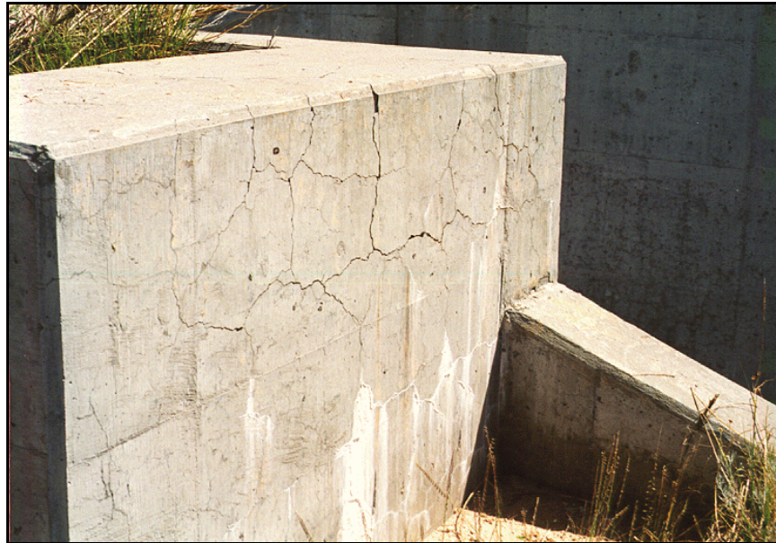
Figure 107. —Concrete deterioration from alkali-aggregate reaction.
