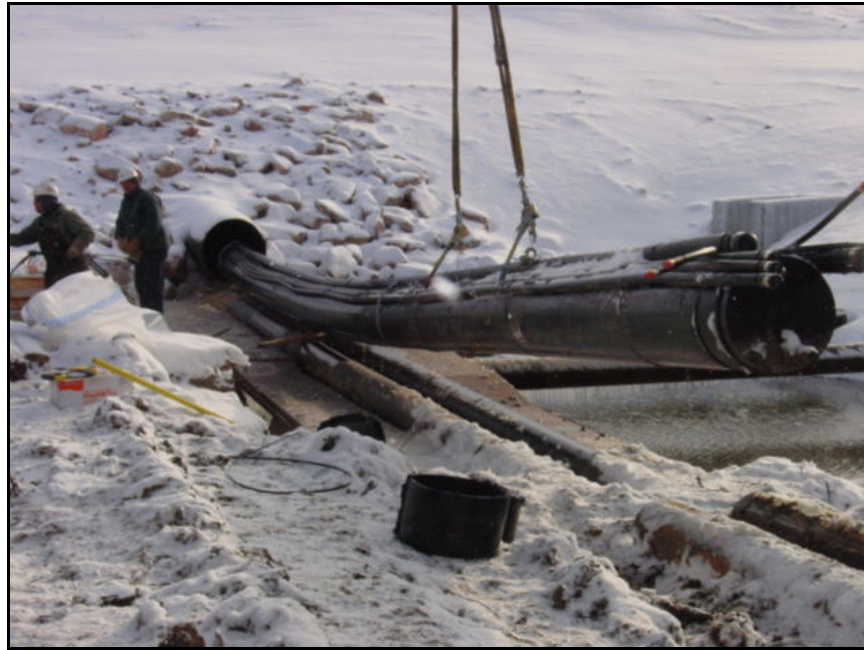
Figure 174. —Insertion of an HDPE slipliner into an existing CMP outlet works conduit.
