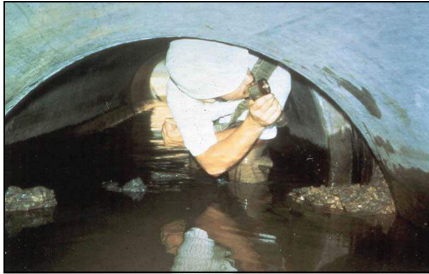
Figure B-49. —The pipe joints separated when foundation movement occurred during construction of the embankment dam.
