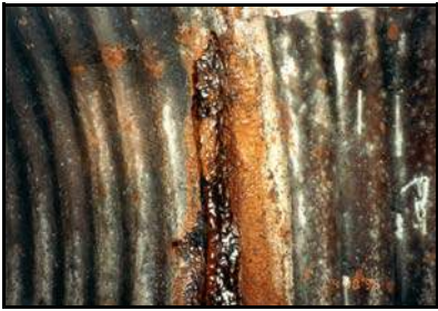
Figure 112. —CMP corrosion within an outlet works conduit caused by a leaking pipe joint.
