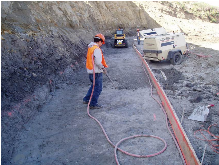
Figure 10.3.1-4 Bonneau Dam Modification, Montana. Foundation cleanup for placement of dental concrete. Rocky Boys Indian Reservation, Montana. USBR 2004
