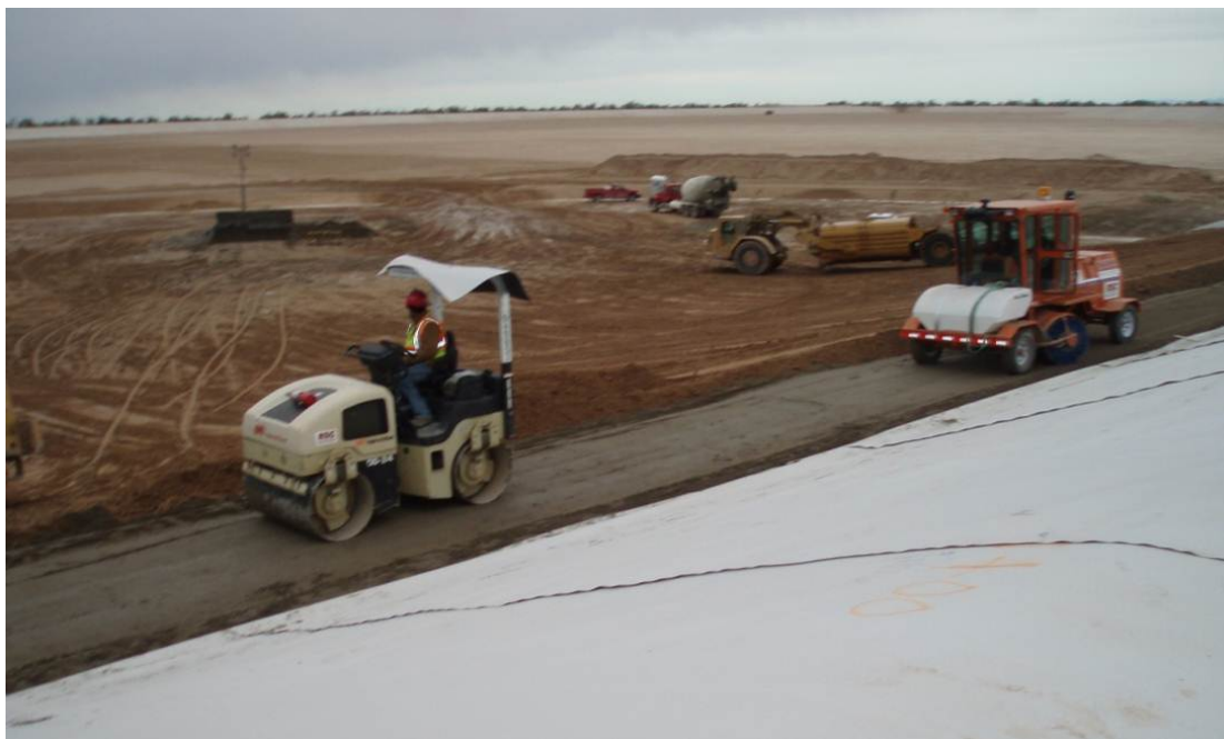
Figure 10.6.8.2.2-1 Warren H. Brock Reservoir, California. Placement of soil-cement on the interior embankment slopes using the plating method (top photo) and stair step method (bottom photo) of placement. USBR 2009
