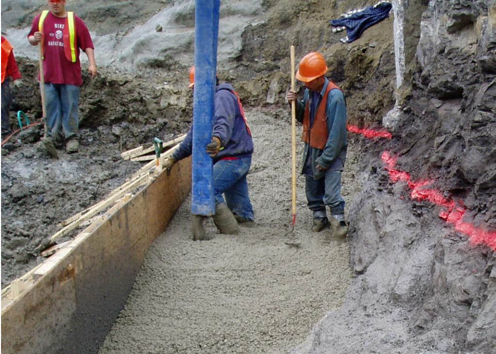
Figure 10.3.1-5 Bonneau Dam Modification, Montana. Protective dental concrete being placed over easily weathered shale to prevent the foundation from weathering. Rocky Boys Indian Reservation, Montana. USBR 2004
