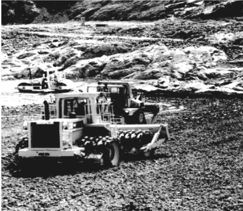
Figure 10.6.3.4-1 A Caterpillar, model 825C, roller compacting impervious fill (zone 1). The roller feet are elongated (chevron feet). Also, notice the filter upstream of zone 1 being compacted by a vibratory roller. The filter is placed over weathered and fractured zones in the foundation rock. USBR, July 1990
