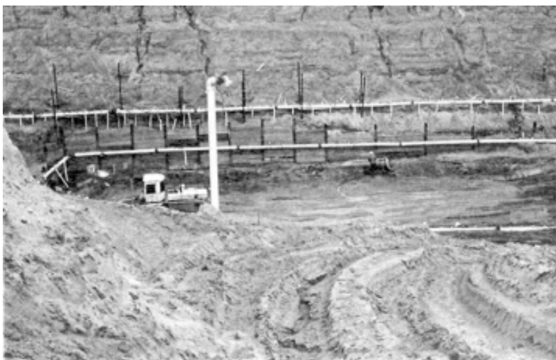
Figure 10.4.1.3-2 Virginia Smith (Calamus) Dam, Nebraska. Multistage well point and deep well dewatering system used for dewatering the stilling basin for the outlet works. USBR 1982
