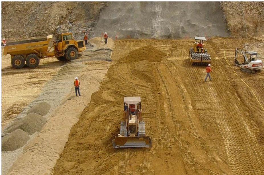
Figure 10.6.1.1-6 Slickrock Creek Dam, Iron Mountain Mine, California. Embankment core material is being spread and compacted. Note that the truck crossing over the sand filter and gravel drain material has a geotextile cover to protect them from contamination. Also, fiber concrete has been placed on the rock abutment visible in the background to prevent seepage transport of the core and sand filter into the abutment rock.
