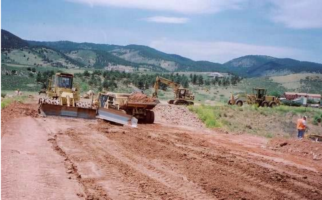
Figure 10.6.3.2-1 Horsetooth Dam Modification, Colorado. Impervious material being dumped, spread by a tracked dozer, and compacted by a tamping or sheepfoot type roller. USBR 2002
