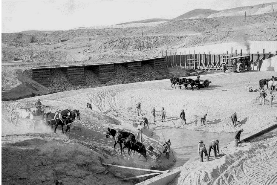
Figure 10.6.1.1-5 The cut and fill method is being used here to construct Lahontan Dam in Nevada, circa 1911. A horse drawn scraper (Fresno) is seen at the bottom center of the picture excavating fill above bedrock, which is being placed on the embankment near the right side of the picture and compacted by a horse drawn compactor. USBR 1911
