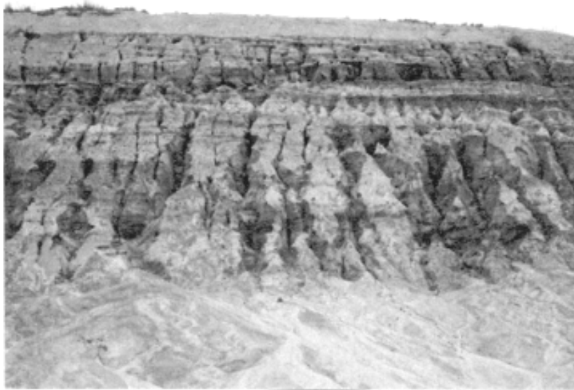
Figure 10.4.1.1-1 Virginia Smith (Calamus) Dam, Nebraska. Erosion of cutoff trench excavation. USBR 1981
