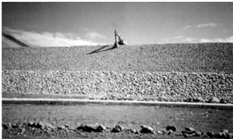
b. Example of excellent results that can be achieved when placing slope protection with a backhoe on the downstream slope of the dam.
