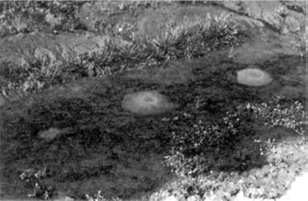
Figure 10.3.1-6 Lake Alice Dam, Nebraska. Sand boils downstream of the embankment near the toe of the dam. USBR 1982
