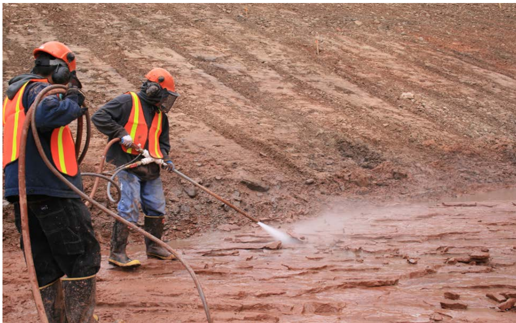
Figure 10.3.1-3 Final foundation cleanup using pressurized air and water to remove loose sandstone and other rock and soil particles.
