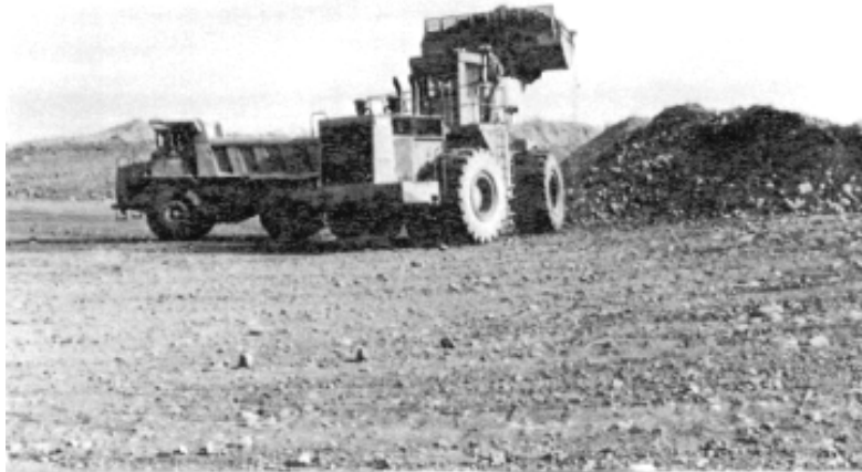
Figure 10.5.1.1.1-1 New Waddell Dam, Arizona. A 12-cubic-yard front-end loader, loading a 30-ton end dump truck with alluvium containing sand, gravel, cobbles, and boulders that will be processed into filter and drain material. USBR 1990
