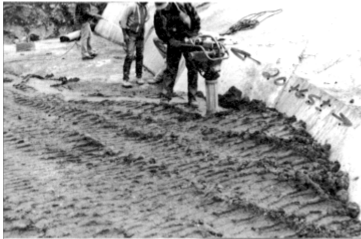
Figure. 10.6.1.2-1 Ridgway Dam, Colorado. Hand compaction along formed dental concrete on an impervious foundation. Notice that this fill has been previously rolled against the foundation by a rubber-tired piece of equipment. The hand compaction is supplemental. USBR 1983
