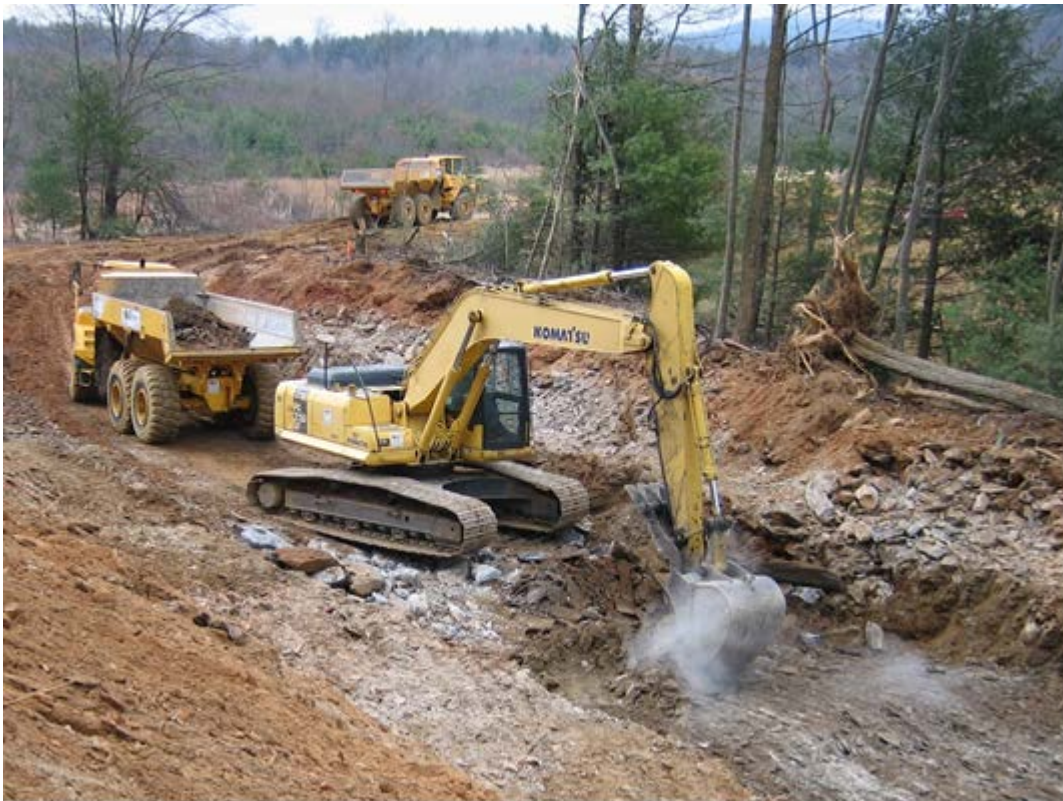
Figure 10.3.1-1 Ore Knob Dam, North Carolina. A back hoe being used to excavate to remove weathered rock. Competent rock is indicated by refusal of the bucket to excavate further. Note the “smoke” (rock dust) being produced by the scraping of the bucket teeth on the hard rock.
