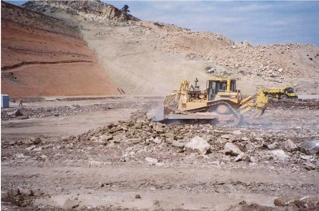
Figure 10.6.1.3.1-1 Dixon Canyon Dam, Horsetooth Dam Modification, Colorado. Crawler tractor spreading a lift of rockfill. USBR 2002
