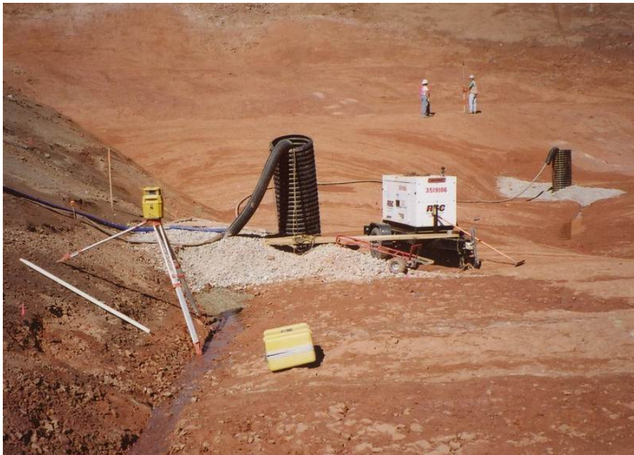
Figure 10.4.1.5-1 Horsetooth Dam, Colorado. Sumps used to dry the foundation for placement of embankment materials on the foundation. USBR 2001
