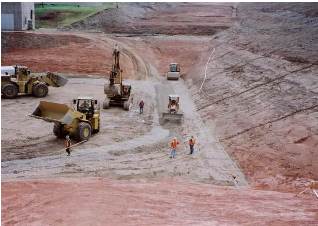
Figure 10.6.4.2-2 Horsetooth Dam Modification, Colorado. Filter compaction by a Cat CS563 smooth drum, vibratory roller, and spreading of drain by a crawler-type tractor. Front-end loaders are being used to haul and dump the filter and drain material.
