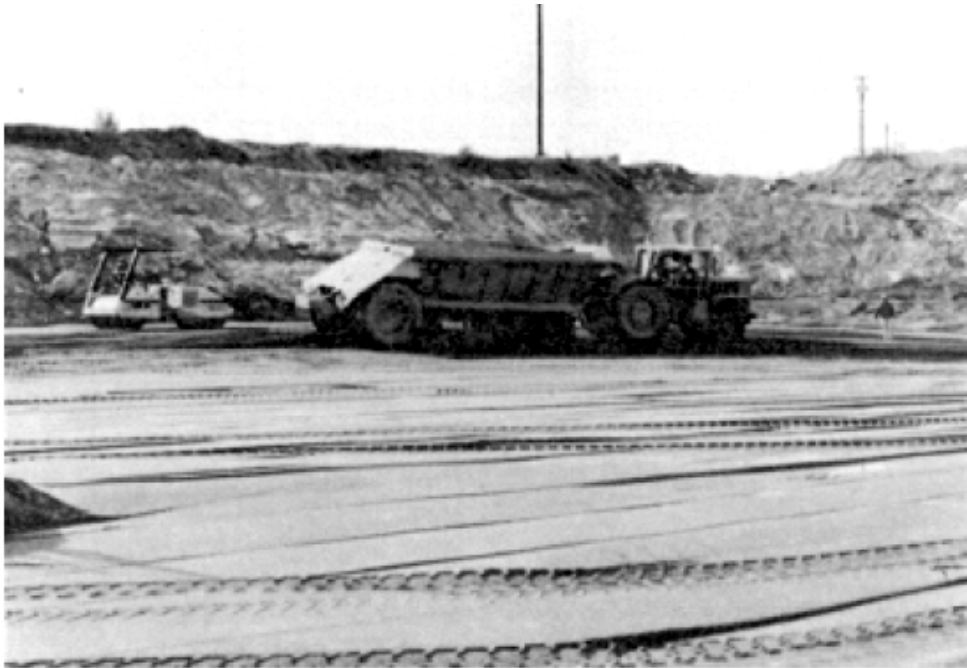
Figure 10.6.4.2-1 New Waddell Dam, Arizona. Bottom dump and 10-ton vibratory roller placing and compacting filter material in the downstream blanket drain. The filter material has been saturated by sprinkling with water.
