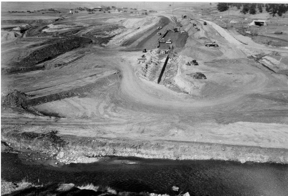
Figure 10.6.7.3-2 Olympus Dam, Colorado. General view looking north at Olympus Dam, which was under construction on the Big Thompson River, showing the river diversion around the south end of the dam. USBR 1947
