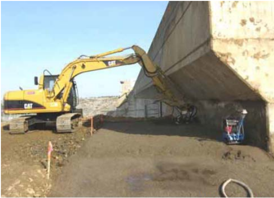
Figure 10.6.4.2-3 Folsom Left Wing Dam, California. View of a sand filter being compacted by a Cat 330L excavator with a vibratory plate compactor attachment. Also notice the hand operated vibratory compactor in the right side of the picture that is used for compacting against the concrete face. This is the interface of the embankment and concrete dam. 2008.
