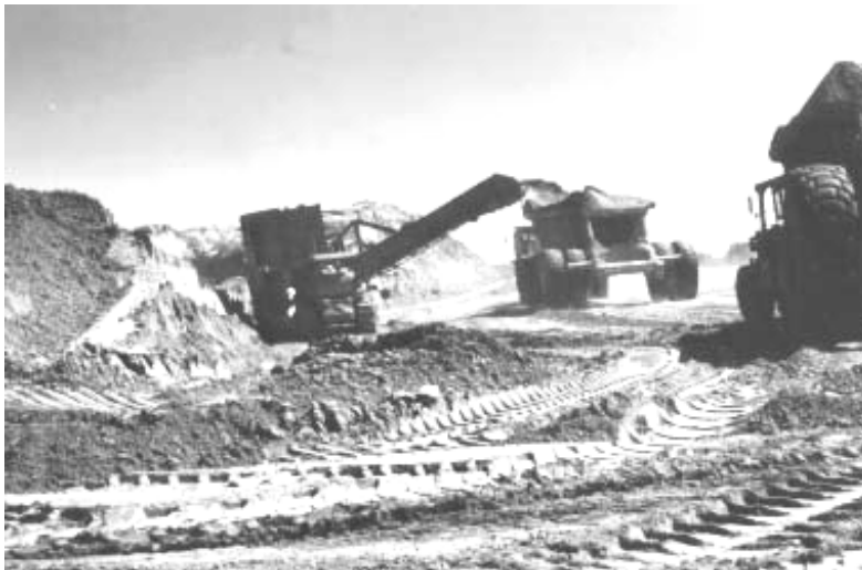
Figure 10.5.1.1.1-2 Virginia Smith (Calamus) Dam, Nebraska. A Holland wheel loader excavating a vertical face mixing silt and fine sand deposits for impervious fill at Reclamation's Virginia Smith (Calamus) Dam, September 1983
