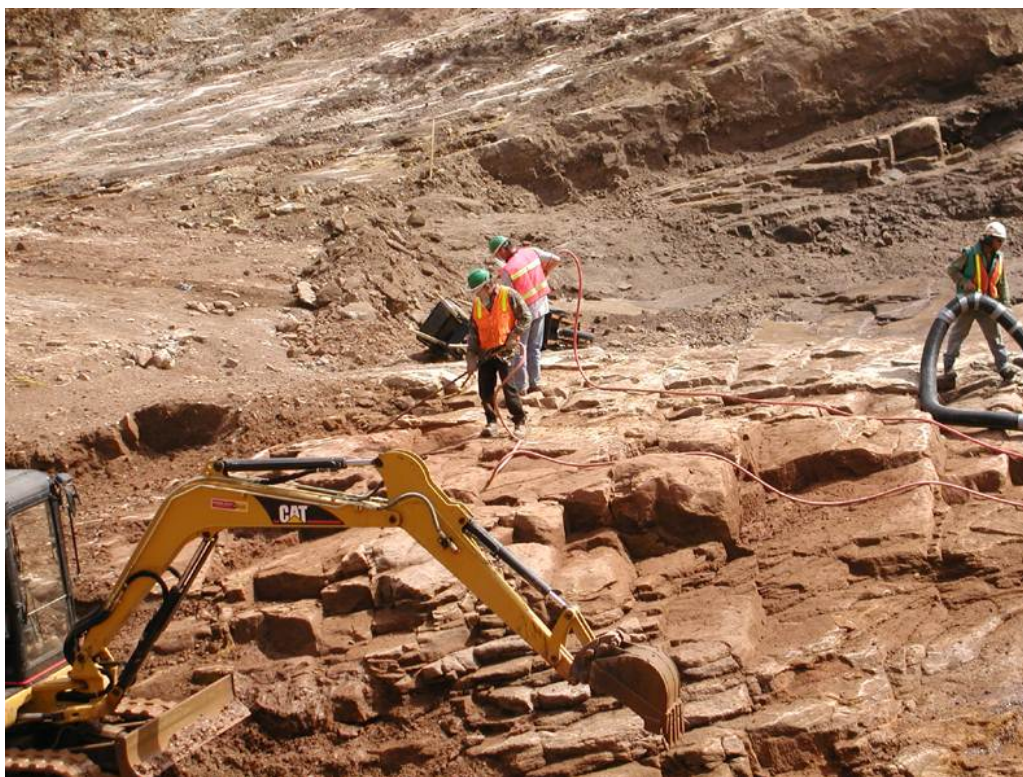
Figure 10.3.1-2 Horsetooth Dam Modification, Spring Canyon Dam, Colorado. Foundation cleanup for placement of embankment materials on the foundation. USBR- 2001-03
