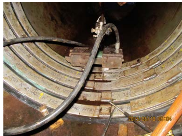
Figure 9. Retaining Compression Bands Locked into Place by a Hydraulic Expander (photo courtesy of NRCS).
