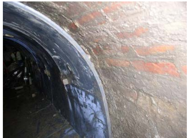
Figure 5. Example of a Mechanical PVC Seal in a Horseshoe-Shaped Masonry Conduit (photo courtesy of Link-Pipe®)
