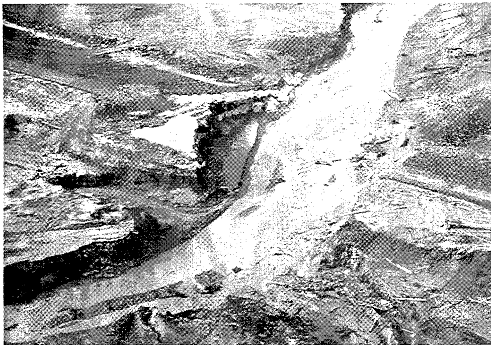
Figure 3. Failed gabion spillway, Toutle River
