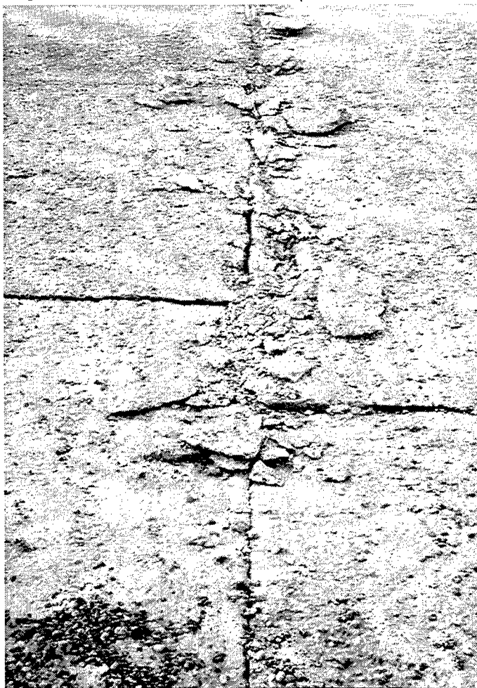
Figure 16. RCC spalling along a joint, Addicks Dam
