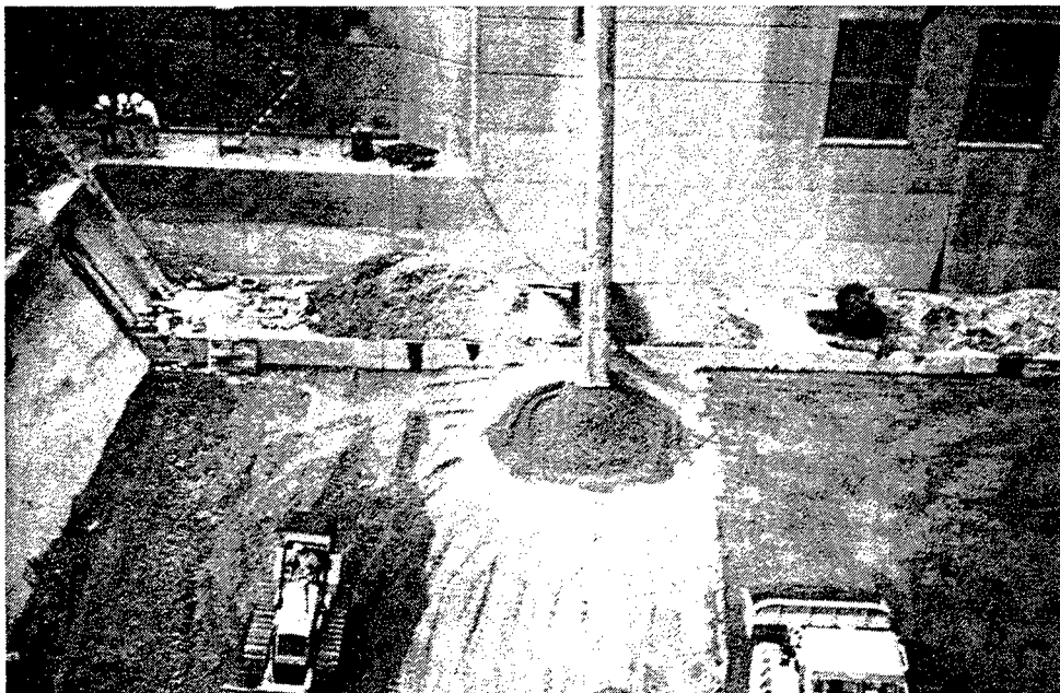
Figure 112. RCC delivered to the lock floor via a drop pipe at New Cumberland Lock (courtesy of Anderson 1984)
