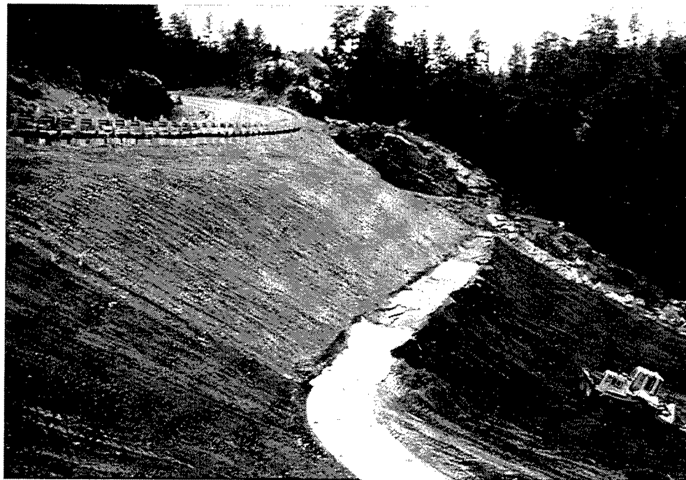
Figure 67. Lift surface covered with blankets and face covered with topsoil, Horsethief Dam
