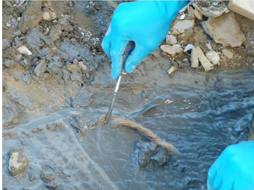
Figure 15.15.3.3-1. Contractor sealing leak by pushing oakum into a crack in sandstone.
