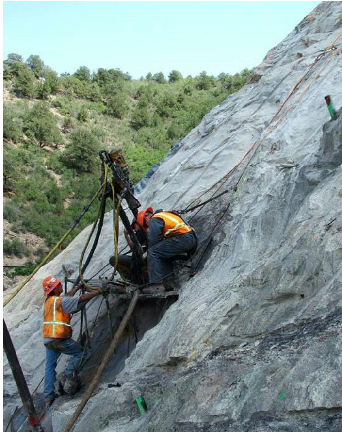
Figure 15.11.2-1. Contractor using a Chicago-pneumatic 65 (CP-65) drill for drilling abutment grout holes on steep terrain.
