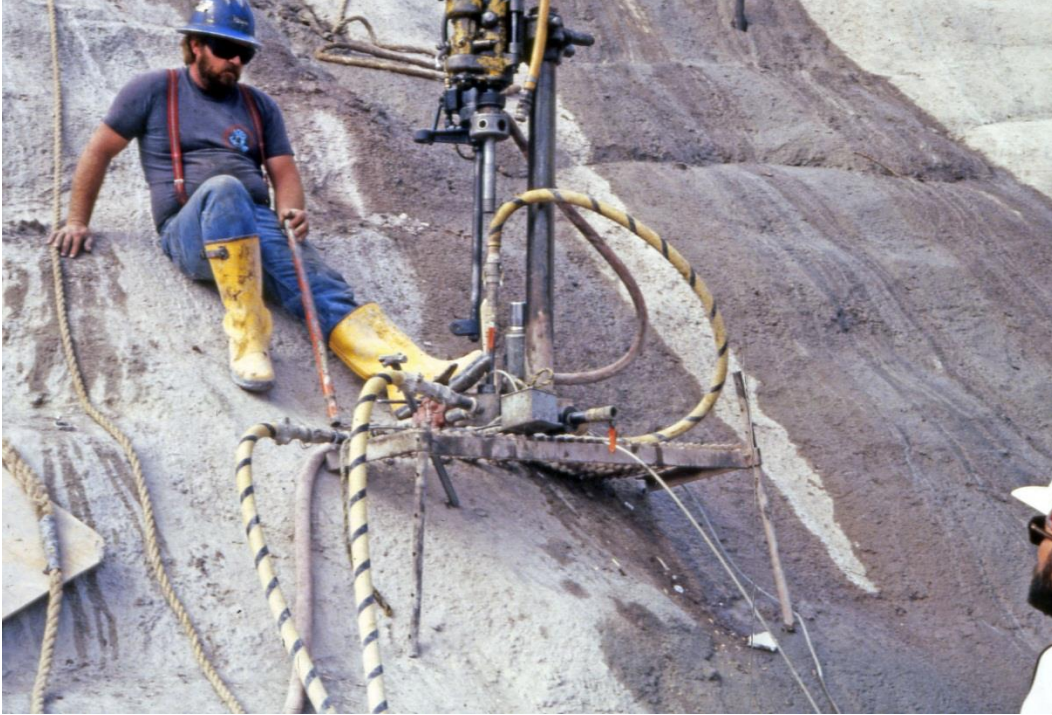
Figure 15.12.7-1. Supply and return grout circulation grout lines at the grout manifold.
