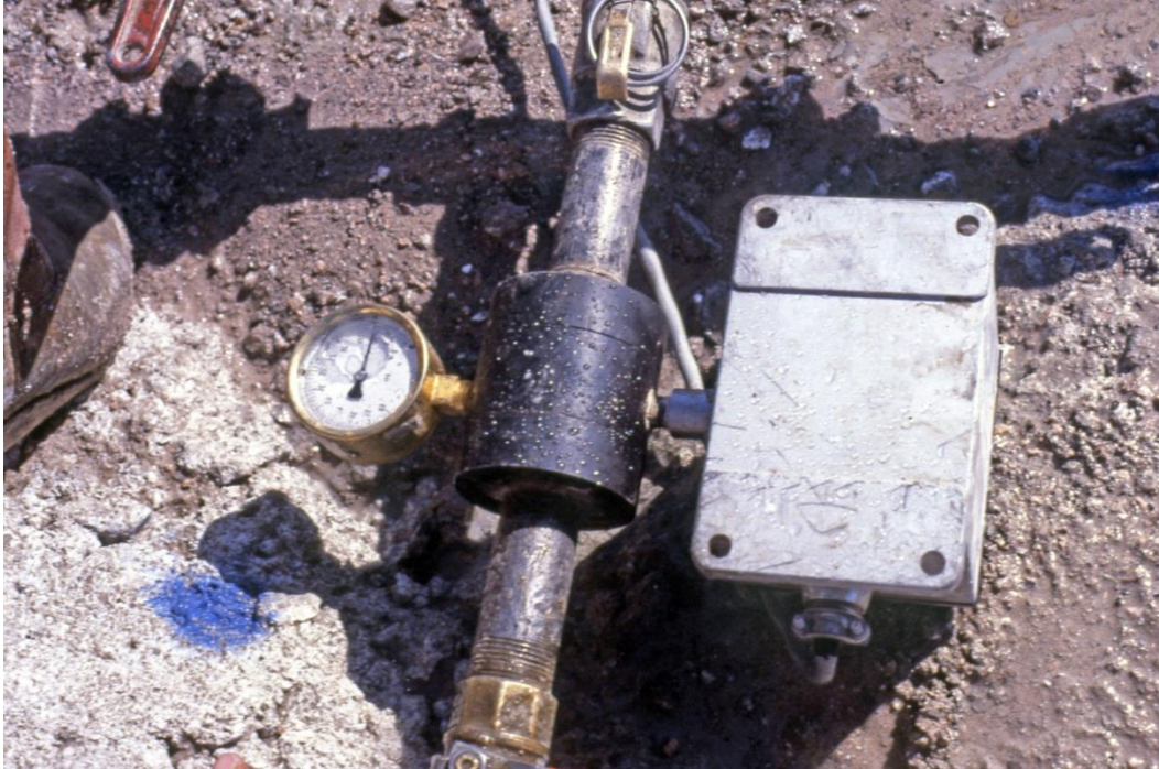
Figure 15.12.6-1. Pressure gauge and pressure sensor on a grout manifold (Series 42 Red Valve pressure sensor).
