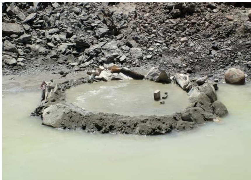
Figure 15.15.3.3-2. This leak has been caulked with oakum and wood wedges. A ring was formed with empty cement bags, earth materials, and grout to apply back pressure and further reduce leakage.
