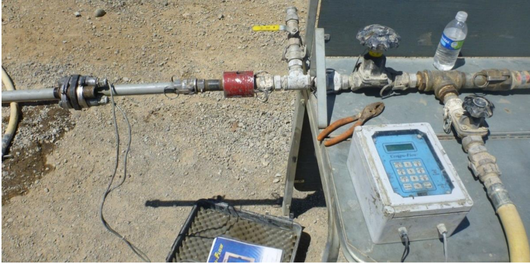
Figure 15.12.9-1. An ultrasonic flowmeter installed downstream of bleeder valve. The standpipe is not shown in the photo.
