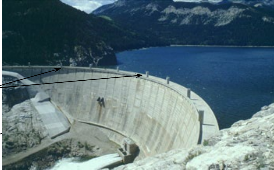
Overtopping protection for concrete dam (rockbolt and mass concrete armorment of right and left abutment and modified dam crest to serve as auxiliary spillway), Gibson Dam, Montana
