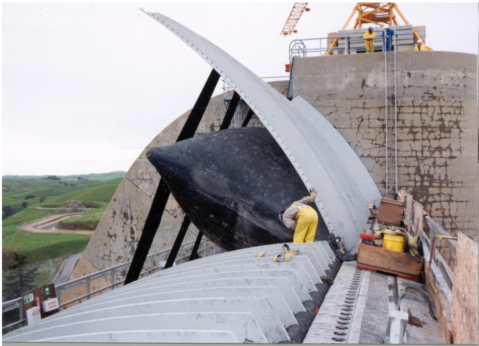
Figure 3.9.1.1-5. Crest gate – Obermeyer type.
