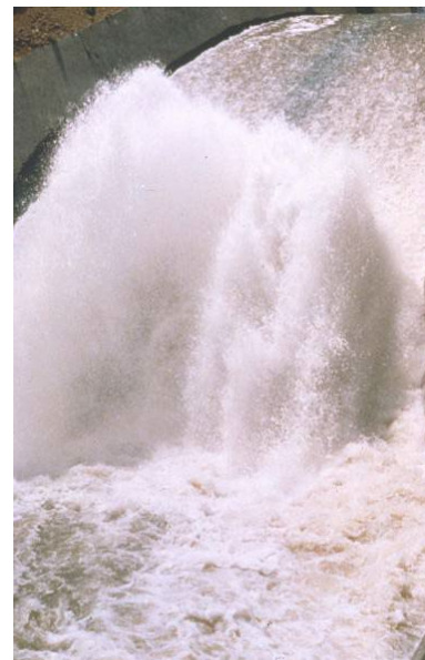
1983 Spillway Chute Damage due to Flood-induced Stagnation Pressure – Big Sandy Dam, Wyoming.
