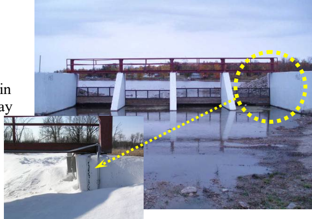
Spillway Walls Fail (concrete walls crack near base and reinforcement yields) due to Frost-Heave – Belcourt Dam, North Dakota
