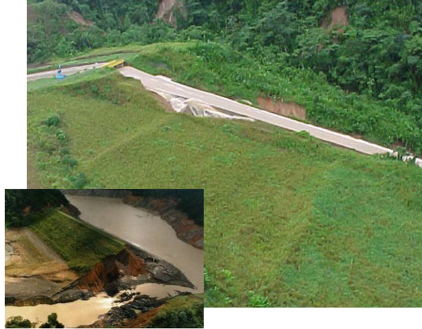
1999 Dam Failure due to Flood-induced Chute Wall Overtopping – El Guapo Dam, Venezuela (courtesy of Ing. Alejandro Hitcher).
