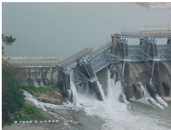
1999 Dam and Spillway Failure due to an Earthquake – Shi-Kang Dam, Taiwan.
