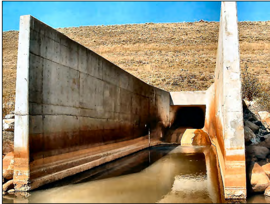
Figure 5.—Hydraulic jump stilling basin. Note the hydraulic jump flow pattern on the interior surface of the basin walls.
