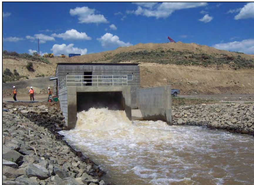
Figure A-22.—View of 42-inch diameter fixed-cone valve discharging at about 20 ft 3 /s.
