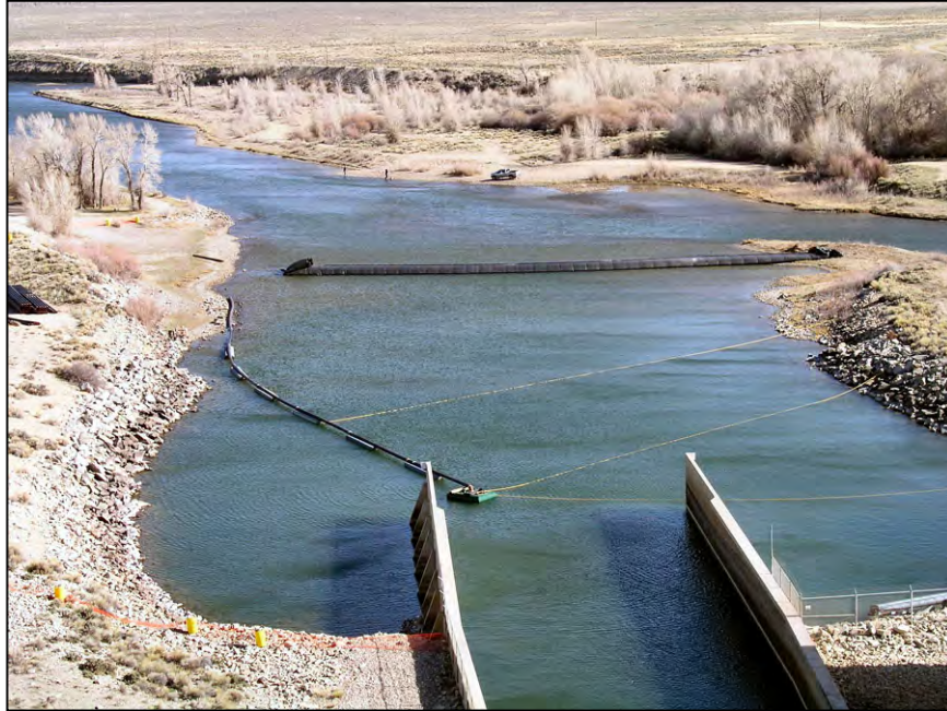
Figure 167. —A polyethylene baffled bladder dam is being placed downstream from a stilling basin. The dam is 250 feet long by 19 feet wide by 8 feet high. The dam weighs 2,600 pounds (dry). Two 3-inch pumps (8 hp) and two 3-inch pumps (4.5 hp) were used to fill the dam with 150,000 gallons of water. The dam took about four hours to deploy (watering up and rolling out the dam). Upon removal, the dam took 2 hours of dewatering and 2½ hours to roll up and remove. Removal of the dam required the rental and use of two track-hoes for rolling up the dam on a log.
