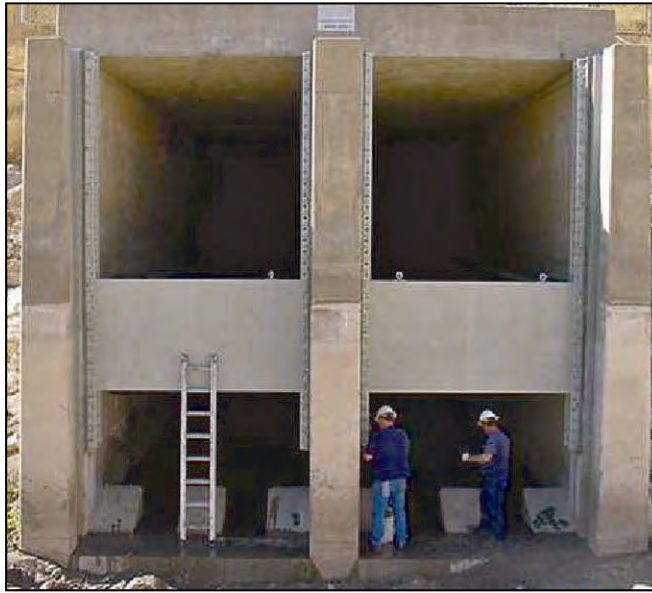
Figure 31. —Flow deflectors being installed at the downstream end of a stilling basin.
