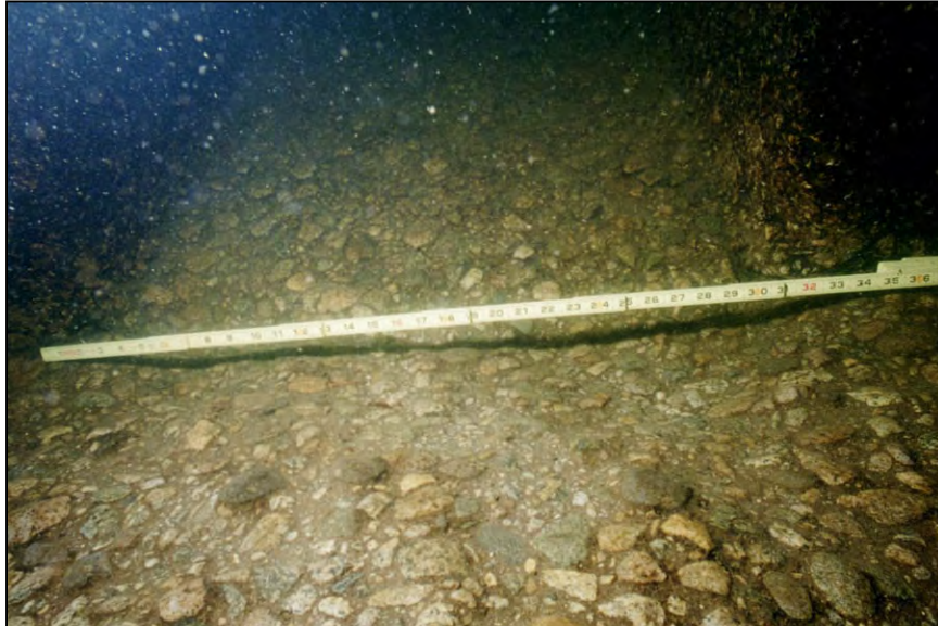
Figure A-115.—Localized erosion between two chute blocks in the outlet works left bay. Note that the ruler is resting on concrete at each chute block and spanning (about 2½ inches above concrete) eroded area in the floor.
