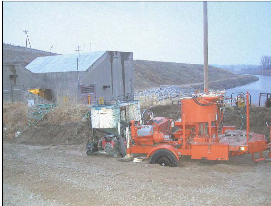
Figure A-127.—Grout pumps located at access road by gate house. White pump was used for grouting and the orange pump was on site as backup pump.
