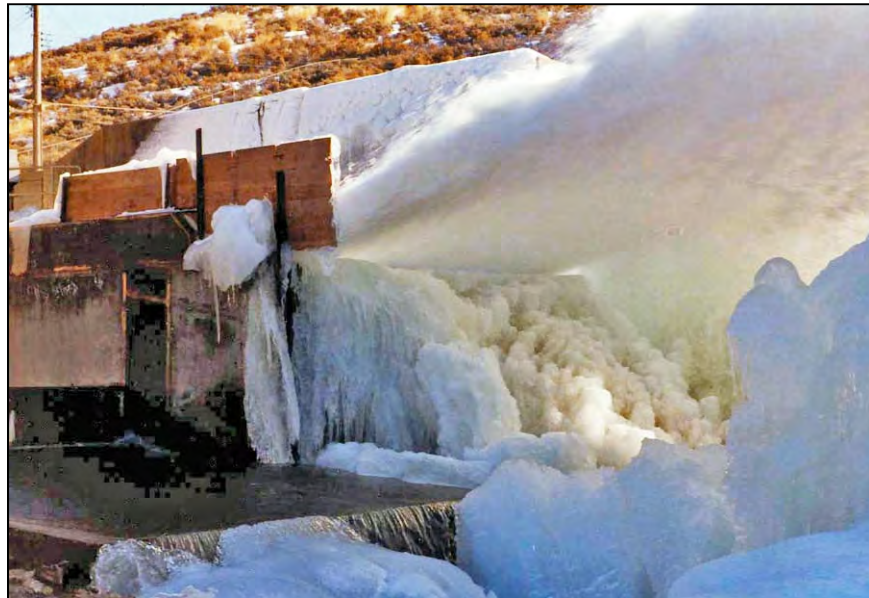
Figure A-46.—Operation of the flip bucket caused significant icing due to water vapor.
