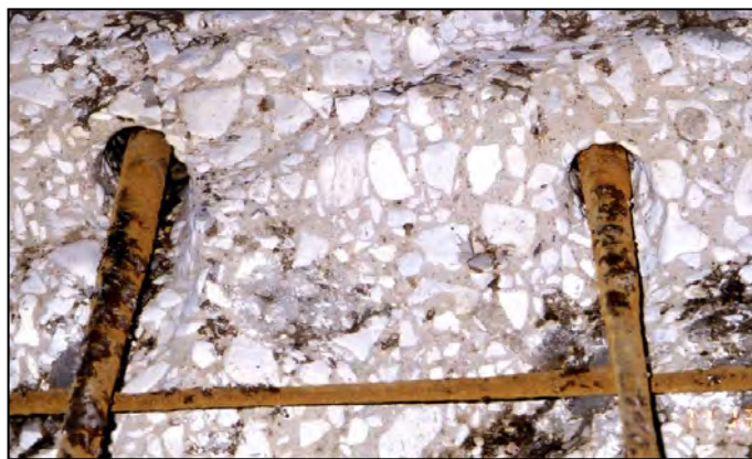
Figure A-122.—Vibration caused the conical openings around the portion of bars remaining in concrete.
