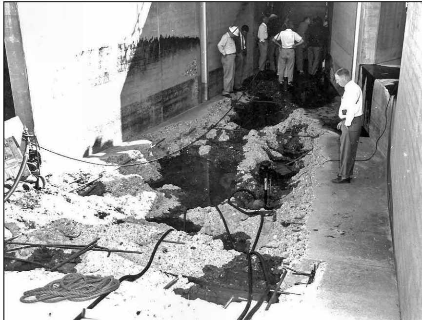
Figure 145.—The invert of this flip bucket sustained significant cavitation damage during operation.
