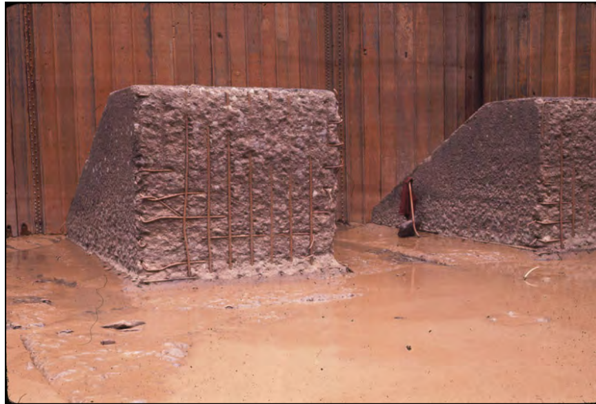
Figure A-39.—Baffle pier damaged by abrasion erosion.
