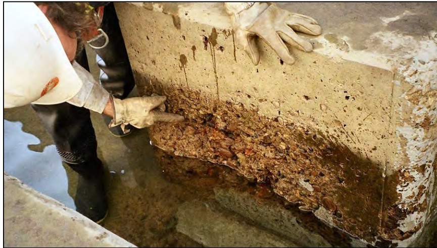
Figure 147.—Abrasion erosion damage at a dentate block.
