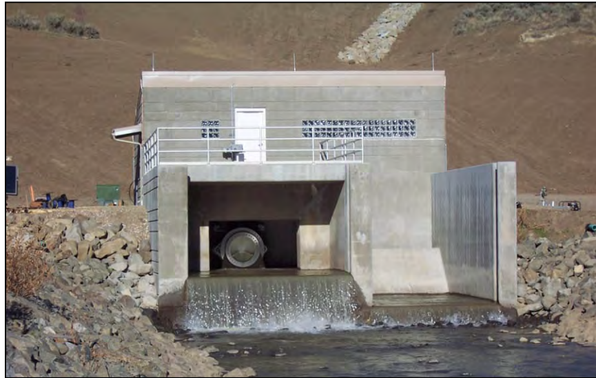
Figure A-21.—View of 42-inch diameter fixed-cone valve under low flow conditions.
