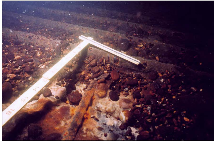
Figure A-14.—View of outlet works stilling basin showing larger exposed transverse rebar and lower longitudinal rebar. Erosion of floor in this area is approximately 6.5 inches. Lack of rust accumulation on rebar indicates active scour of basin floor.
