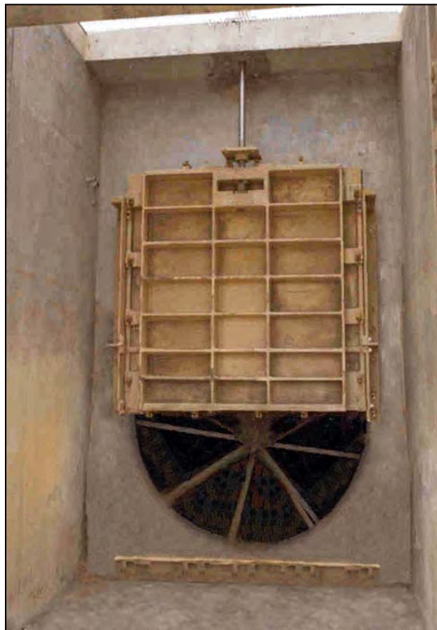
Figure 104.—Unbonneted slide gate.
