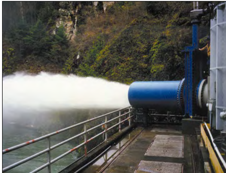
Figure 97.—Jet-flow gate in operation. Photo courtesy of URS Corporation.
