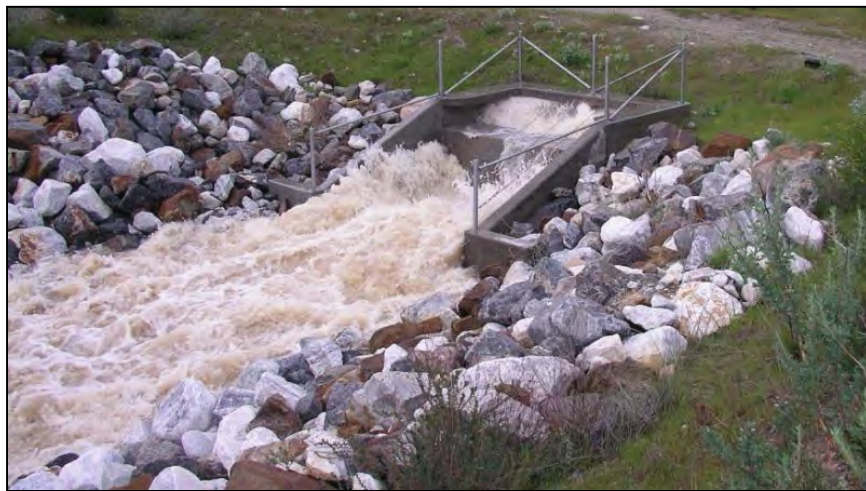
Figure A-93.—Same energy dissipator with flow (120 ft 3 /s).
