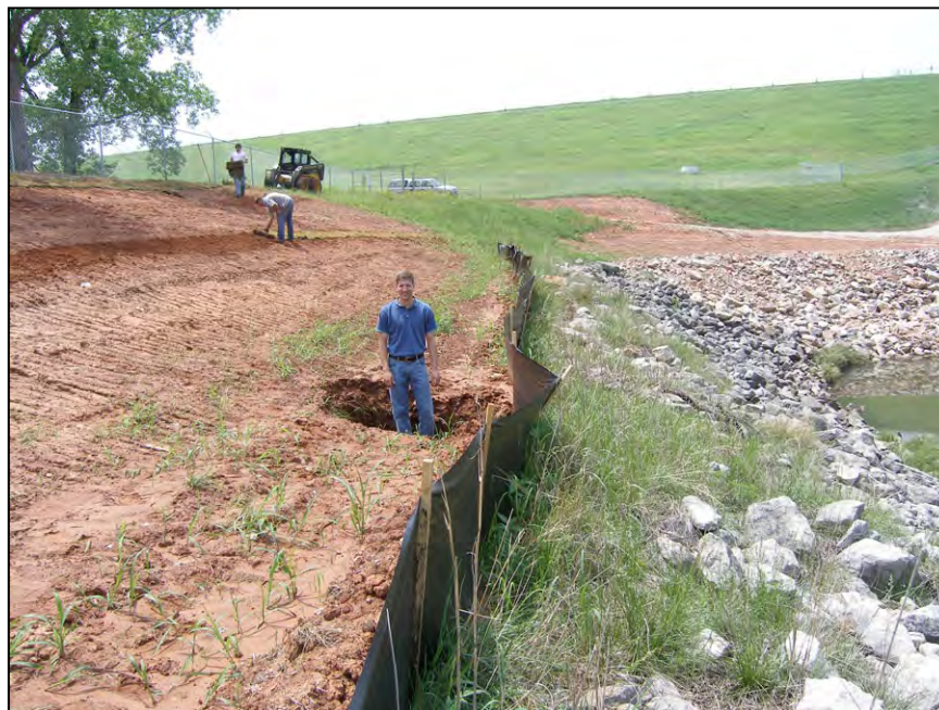
Figure A-66. —After the basin was refilled, a sinkhole approximately 3 feet deep and 3 feet wide appeared on the surface of the bank above the water line.
