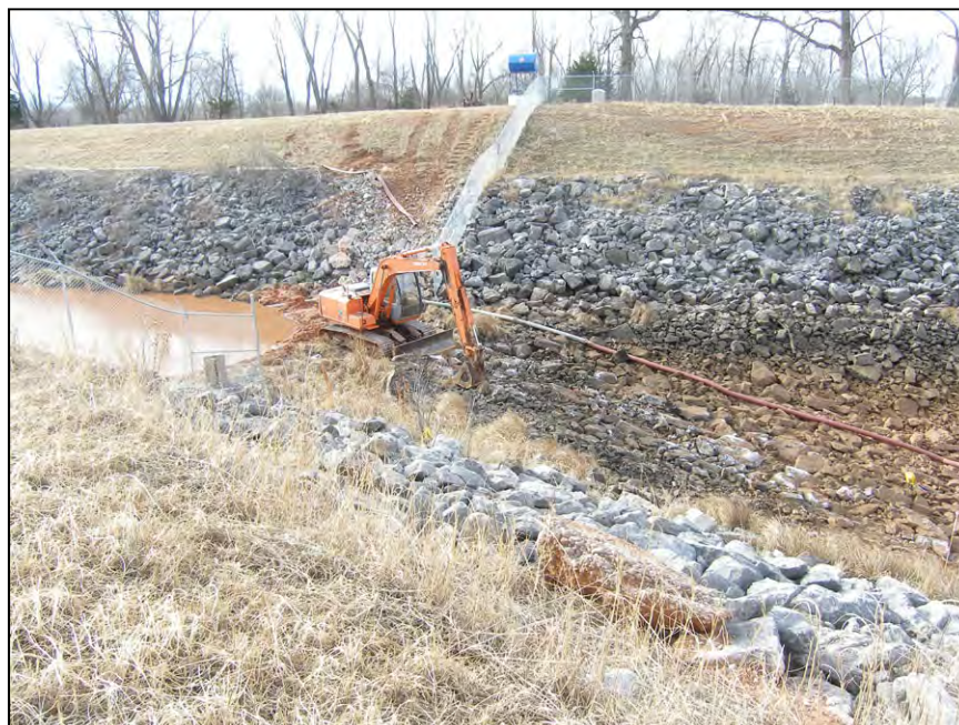
Figure A-60.—The contractor created a small earthen dike in the downstream river channel to facilitate unwatering of the stilling basin.
