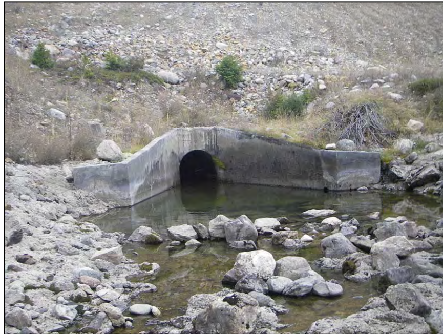
Figure 126. —The grouted riprap has performed well although some of the larger rocks in the foreground are displaced immediately downstream of the concrete apron.
