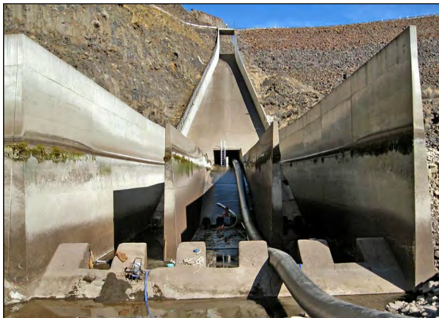
Figure 23.—A dentated end sill for a combined outlet works and spillway stilling basin.
