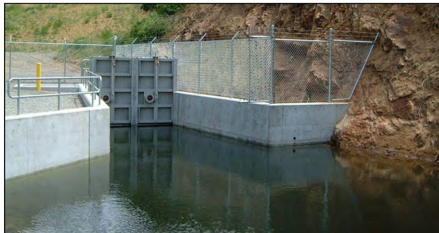
Figure 176.—Fencing at a stilling basin. The steep cliffs also provide an access deterrent.
