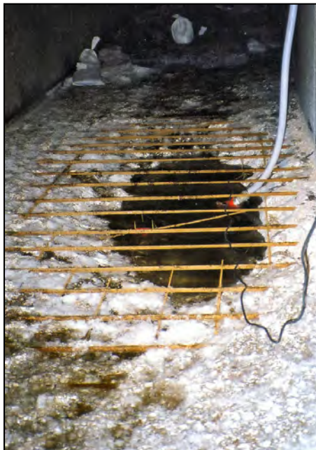
Figure A-121.—Abrasion erosion which occurred on the basin floor.
