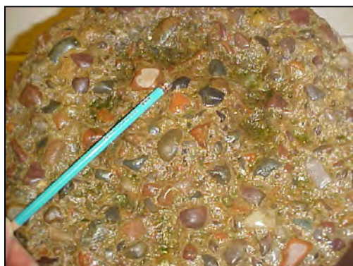
Figure 177.—Minor abrasion erosion damage.
