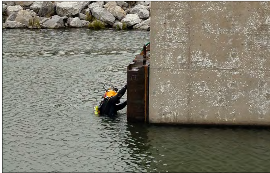
Figure 165.—Divers assisting with the installation of stoplogs at the downstream end of a stilling basin. Turnbuckles were attached to the stoplogs and basin. These held the stoplogs against the end of the basin walls until the basin was unwatered and the outside water pressure kept them in place. Rubber seals on the stoplogs prevented leakage.
