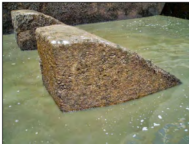
Figure 22.—Baffle blocks in a hydraulic jump stilling basin (flow is from left to right).
