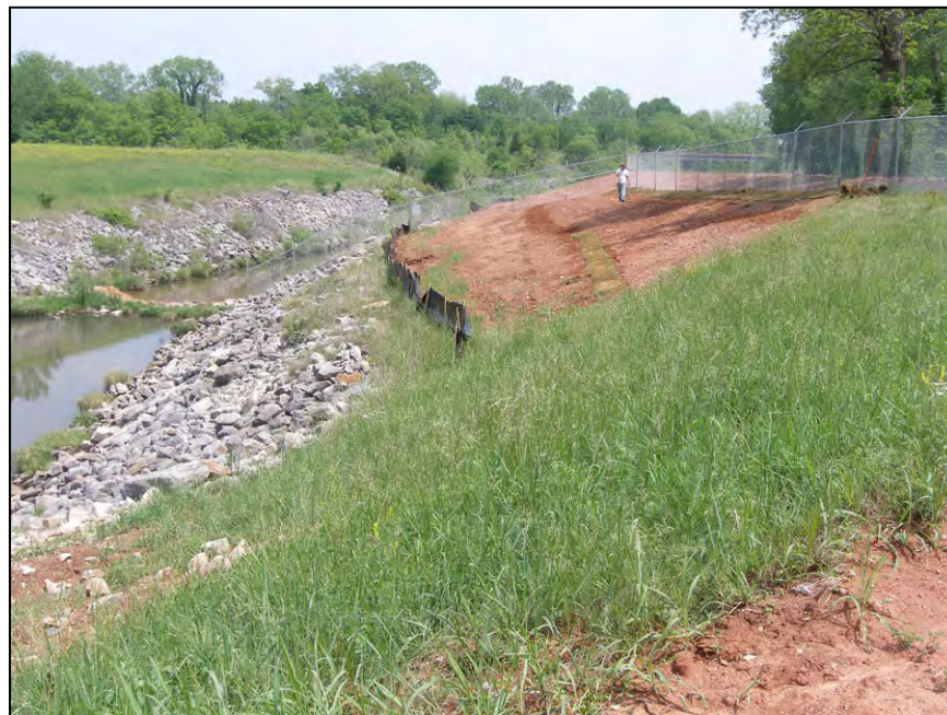
Figure A-65.—Slump area after cutting back slope. Sod is being placed to prevent erosion.
