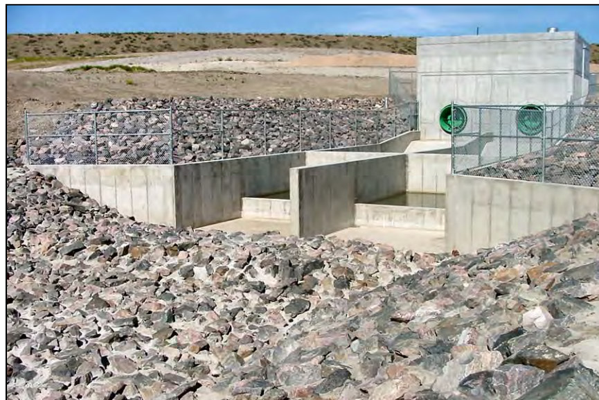
Figure 60.—Concrete-lined plunge basin with baffle wall, grouted riprap side slopes, and discharge channel. Flow discharges into the plunge basin from two 36-inch diameter fixed-cone valves.
