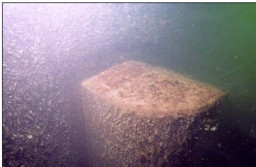
Figure A-13.—View looking downstream at far left dentate showing the general condition of outlet works stilling basin dentates. All dentates were in good condition with well defined edges and corners. No chipping of edges was noted.
