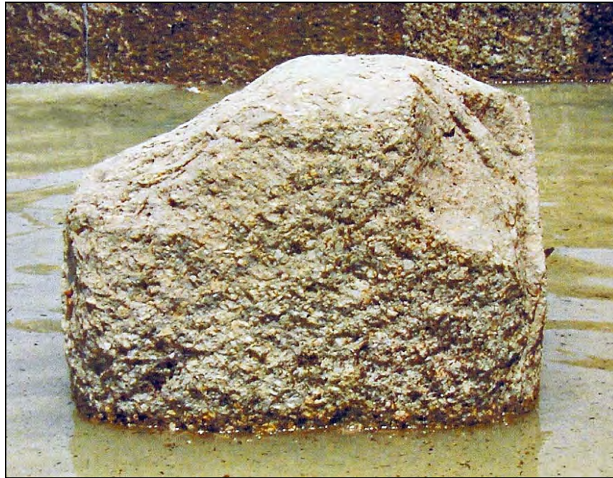
Figure 169. —This baffle block has experienced impact damage resulting from an object in the flow.
