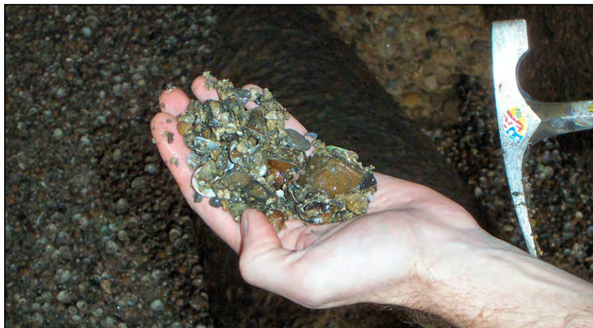
Figure 148.—Eroded concrete caused by abrasion.
