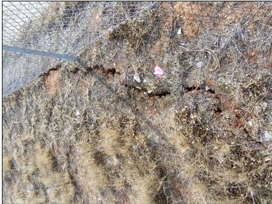
Figure A-64.—Cracking developing on slope near fence line.
