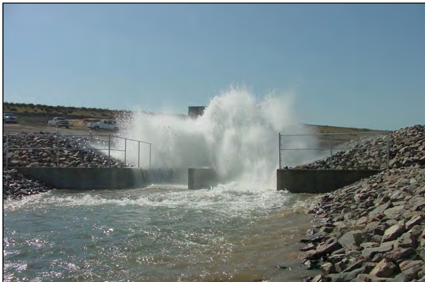
Figure A-102.—View looking upstream at the stream release facility with both fixed-cone valves operating each at 20 percent opening (total of 167 ft 3 /s).
