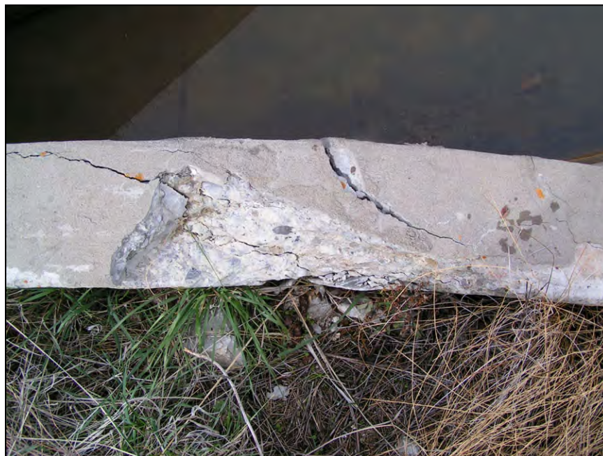
Figure A-57.—Deflection in left wall of dissipator.
