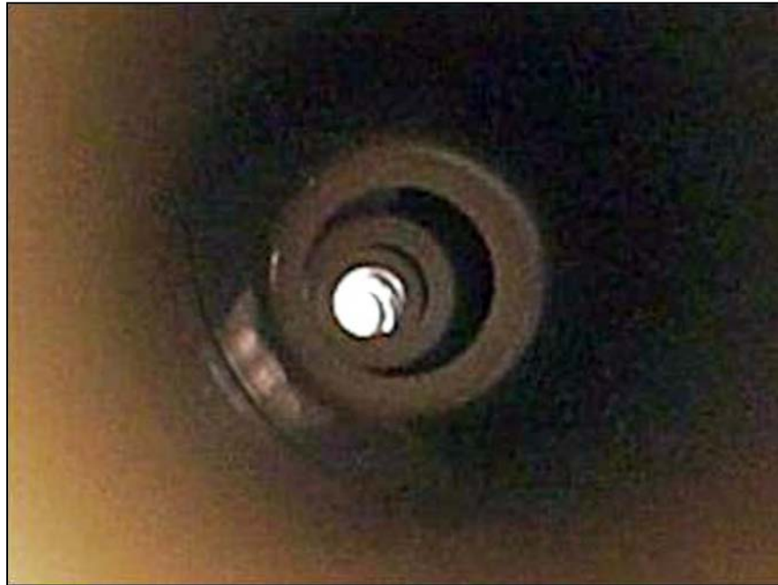
Figure 116.—Looking upstream at inline orifices within a 36-inch outside diameter pipe.
