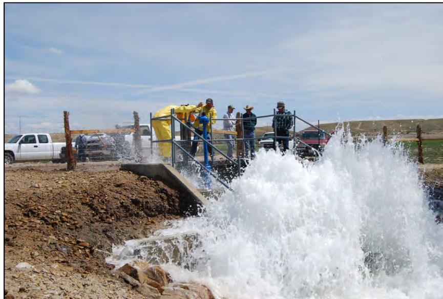
Figure 54. —The end of this outlet conduit was constructed too close to the vertical hanging baffle resulting in intense sprayback.
