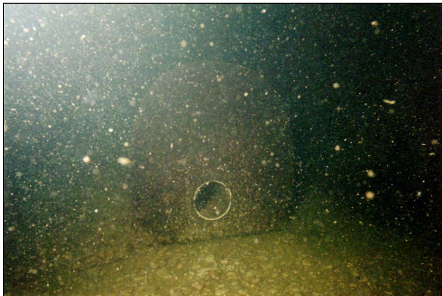
Figure A-106.—Typical condition of downstream face of outlet works stilling basin chute block and 6-inch diameter PVC drain outfall.
