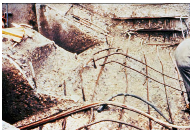
Figure 178.—Severe abrasion erosion damage.
