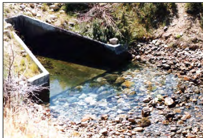
(c) Minor scour exists downstream from the structure after sustained discharge of 270 \text{ ft}^3/\text{s} .
