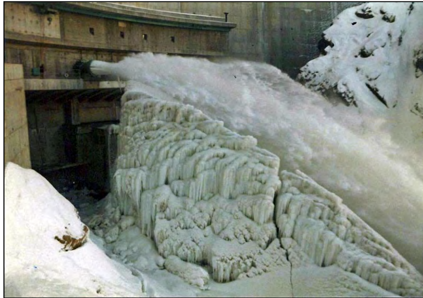
Figure 76.—Ice build-up under 48-inch diameter hooded fixed-cone valves. Ice has built to the elevation of the bottom of the valve operating deck, approximately 60 feet above streambed. Photo courtesy of Denver Water.
