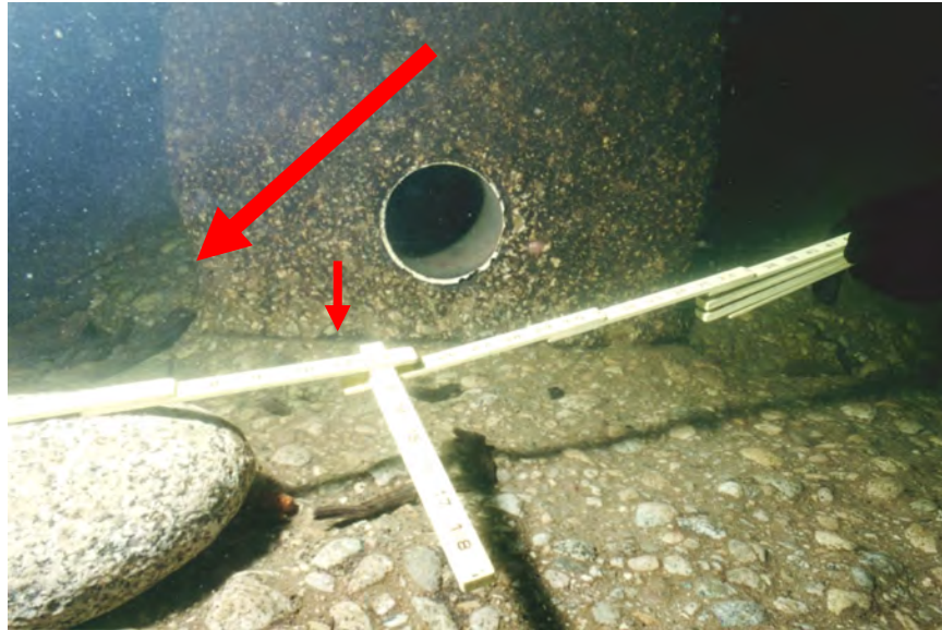
Figure A-114.—Cobble located in left outlet works bay near chute block. Large arrow indicates location where erosion of downstream corner/edge of chute block and floor slab are visible (Note joint along base of chute block at original floor slab denoted by small arrow).
