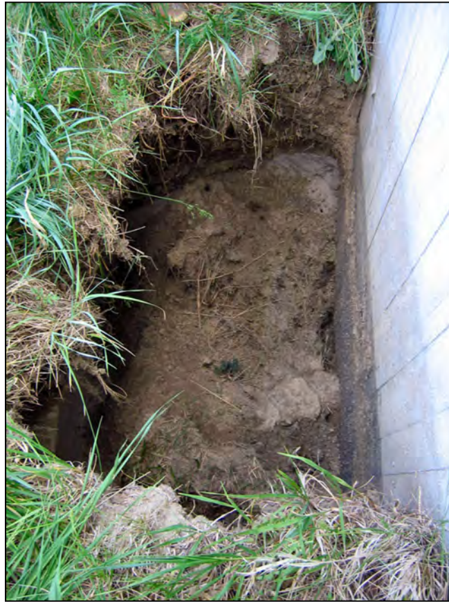
Figure 154. —A sinkhole developed next to this basin wall indicating internal erosion of foundation materials was occurring.
