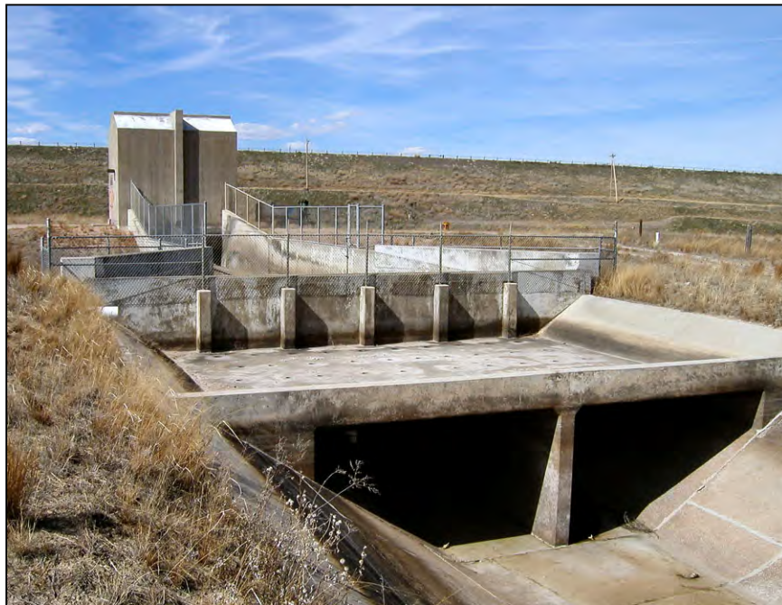
Figure 34. —This wave suppressor (also known as an underpass-type) was constructed after completion of the stilling basin to prevent unanticipated waves exiting the basin from overtopping the downstream canal lining. Overtopping could result in either undermining of the soil supporting the canal lining or introduction of uplift pressures beneath the canal lining. Note the formed openings through the deck of the wave suppressor.
