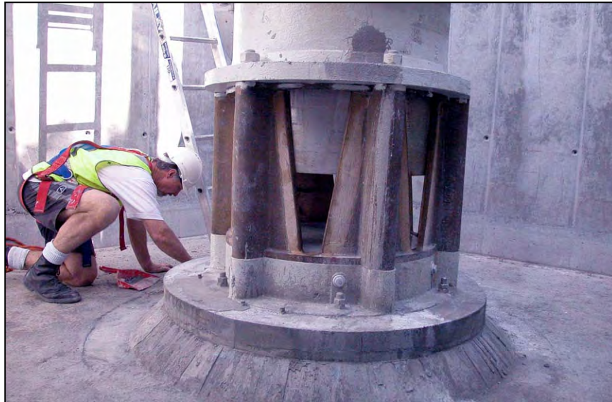
Figure 91. —Bottom discharge of a submerged discharge valve. Note the V port openings.
