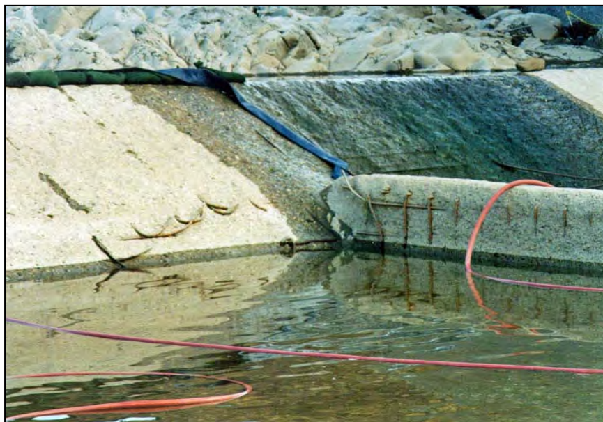
Figure A-70.—Damage to dentate sill.
