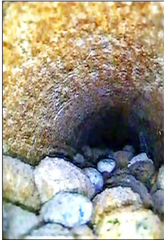
Figure A-112.—Typical condition of Underdrain Nos. 2 and 3 downstream of the second bend, where camera could no longer be advanced.
