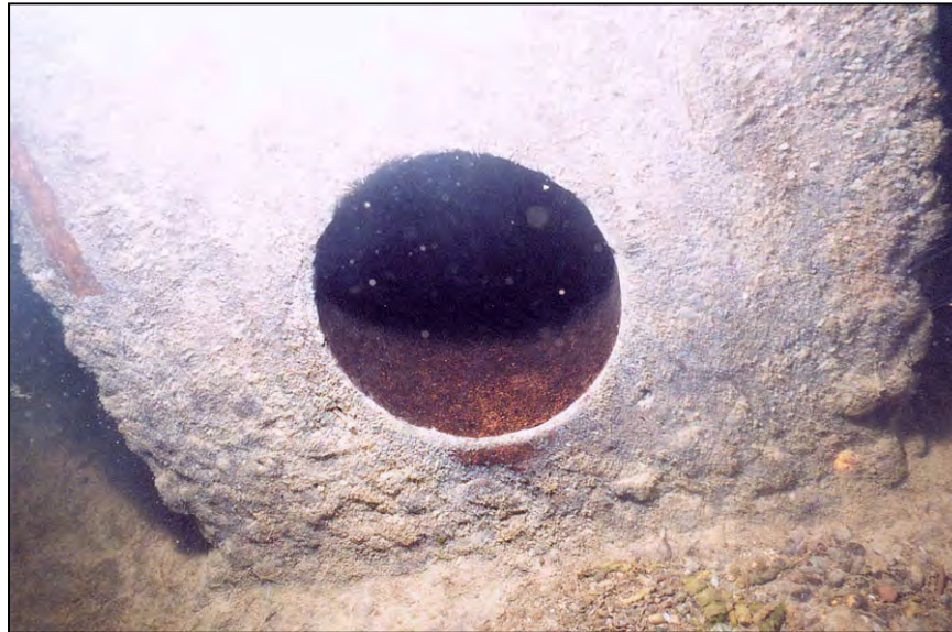
Figure A-11. —View looking upstream at outlet works stilling basin left chute block underdrain. The drain is clear and flowing. Note edge relief of the chute block and the exposed vertical rebar on the left side of block. Concrete erosion of block is approximately 1.5 to 2 inches.
