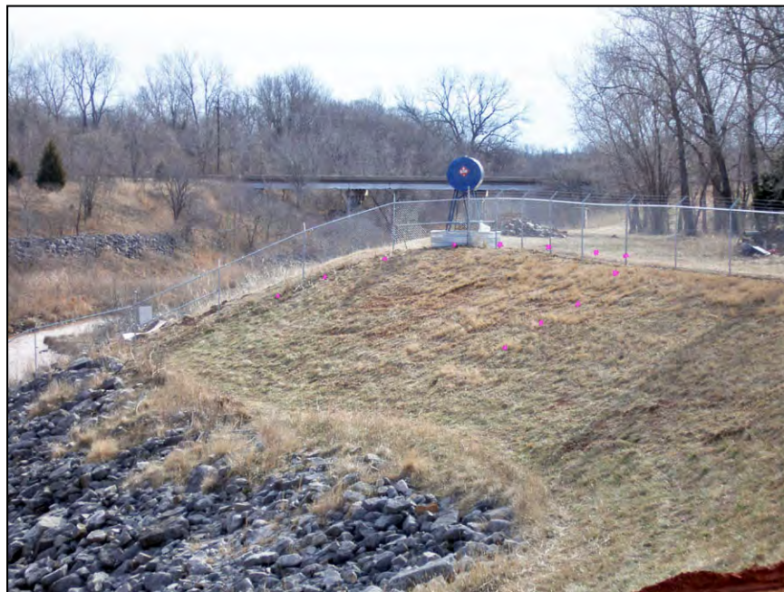
Figure A-63.—Shortly after unwatering, an excavated slope downstream and to the right of the stilling basin was observed to be experiencing cracking and developing a slump. There are pink flags marking the edge of the slump area.
