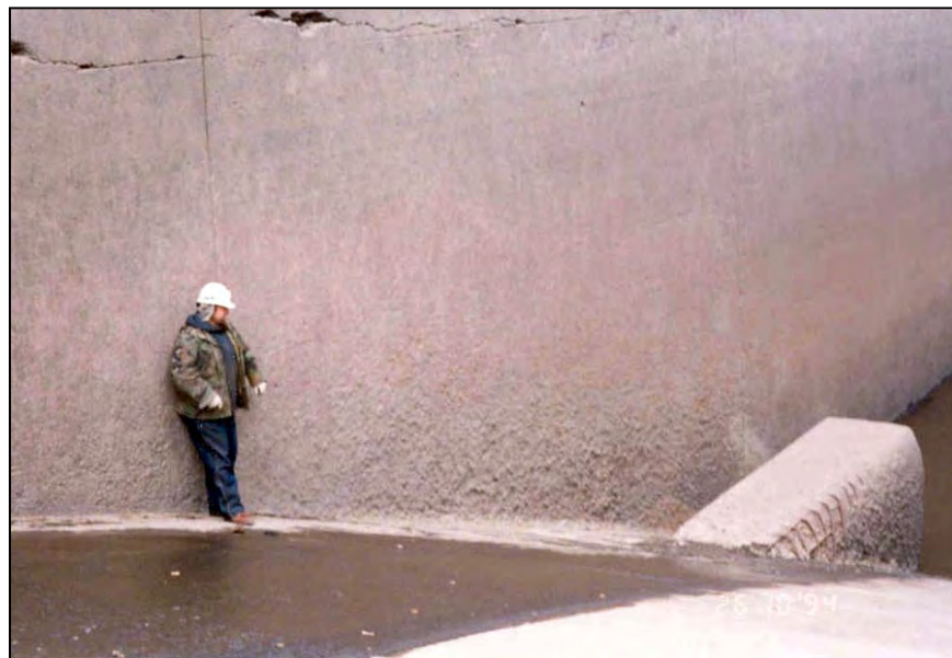
Figure A-68.—Damage to chute block. Note the exposed reinforcement.
