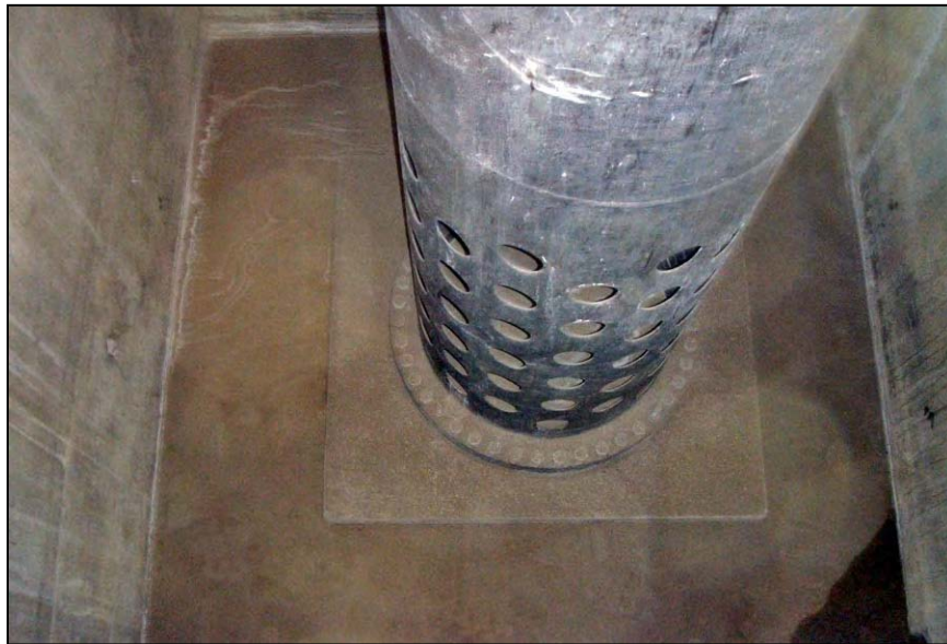
Figure 9.—This 48-inch diameter perforated steel discharge pipe is located downstream of the sleeve valve in a stilling well. The 72 6-inch diameter openings are provided to more evenly distribute the flow from the sleeve valve into the well. The stilling well dissipates any remaining head after the sleeve valve and releases water into the downstream chute without any spray that may cause icing.
