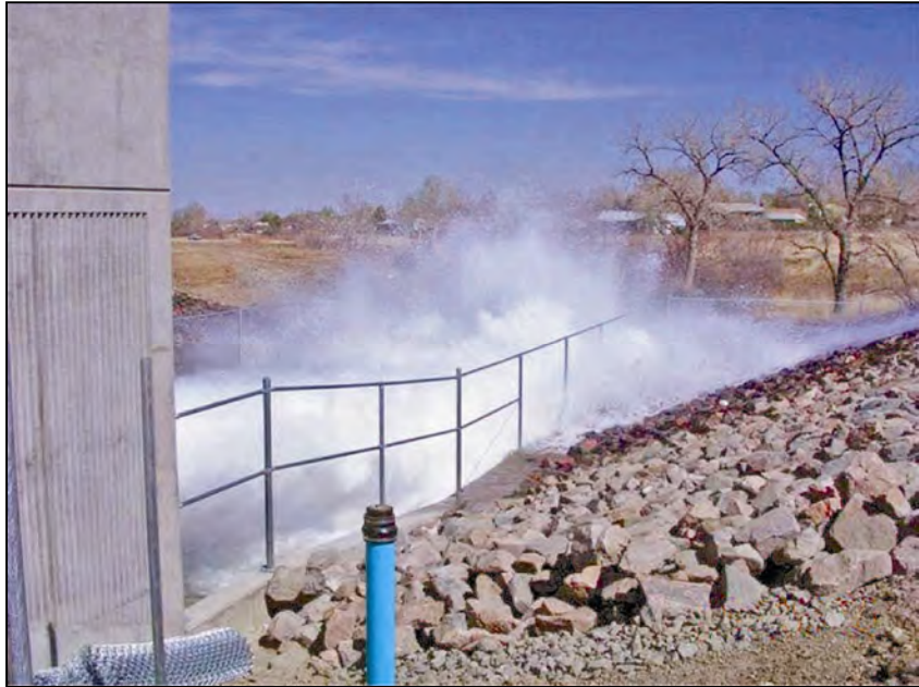
Figure A-100.—View looking downstream shown the right fixed-cone valve discharging at 35 percent opening ( 150 \text{ ft}^3/\text{s} ).
