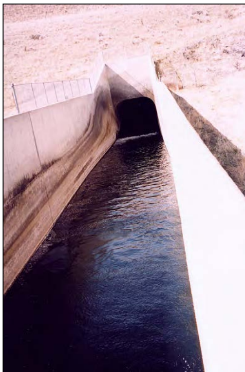
Figure A-10. —View looking upstream at the outlet works stilling basin. During the inspection of the basin, approximately 25 ft 3 /s was flowing through the outlet works.
