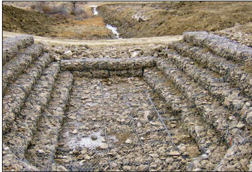
Figure 127. —Gabion-lined basin. The earthen basin was used to facilitate construction access and has been removed.
