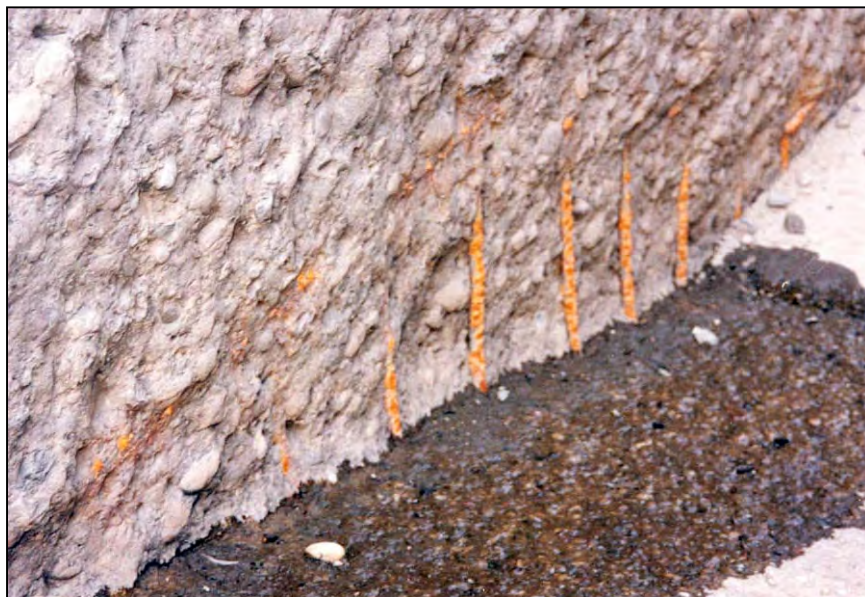
Figure A-69.—Damage to splitter wall.
