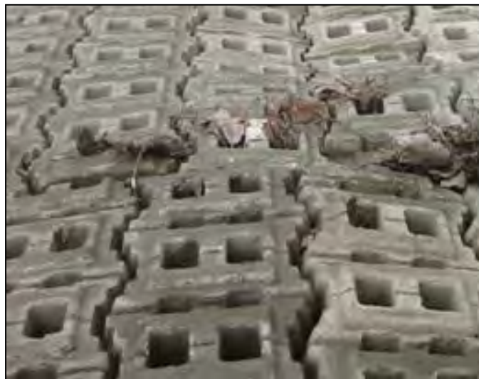
Figure A-33.—Abraded concrete block surfaces.
