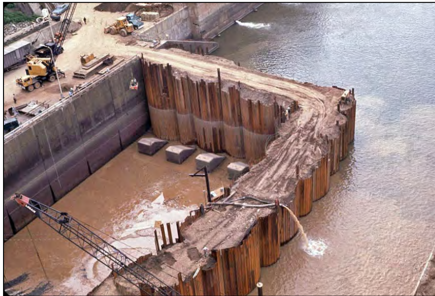
Figure A-38.—Abrasion erosion of stilling basin slab. Note the constructed cellular cofferdam that encloses a portion of the basin.
