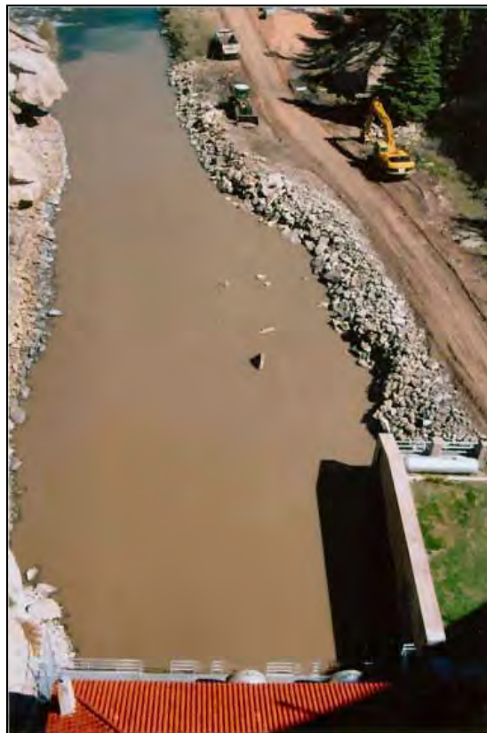
Figure 83. —A 48-inch diameter hooded fixed-cone valve. Note erosion of riprap in downstream channel. Photo courtesy of URS Corporation and Denver Water Board.
