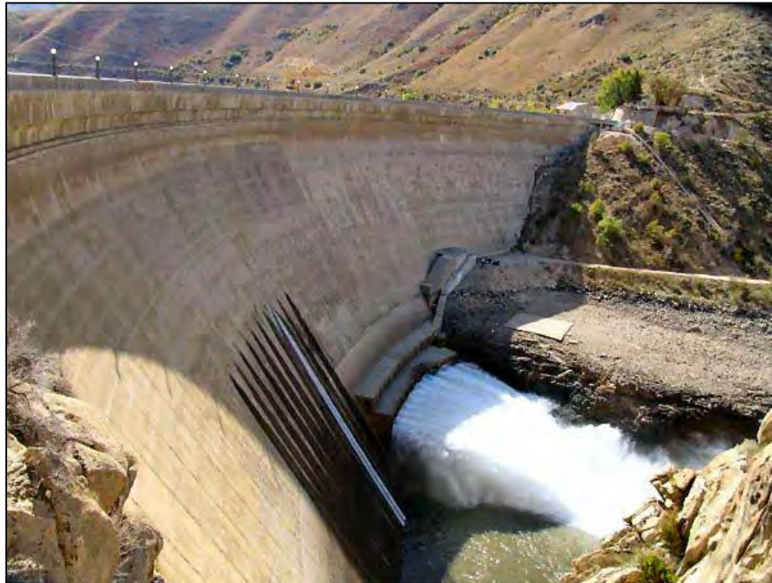
Figure 110.—Ten clamshell gates operating fully open.
