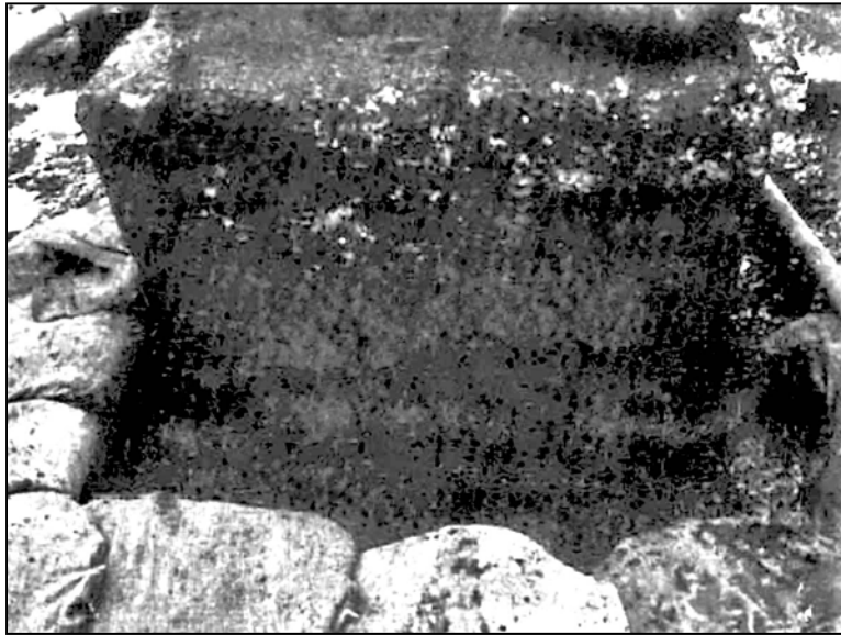
Exposed reinforcement at base of baffle
