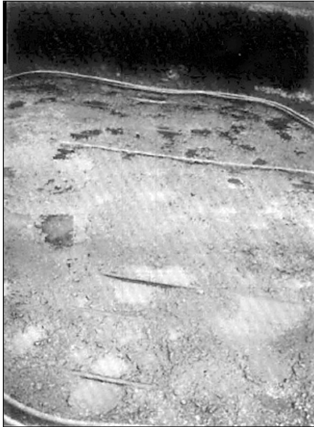
Figure A-8.—Exposed reinforcement in the stilling basin downstream of the baffles.
