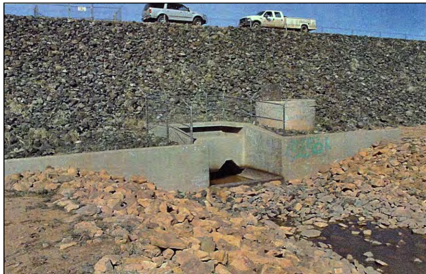
Figure A-27.—View looking upstream at the completed outlet works stilling basin and discharge channel. The structure just to the right of the stilling basin is a toe drain inspection well.
