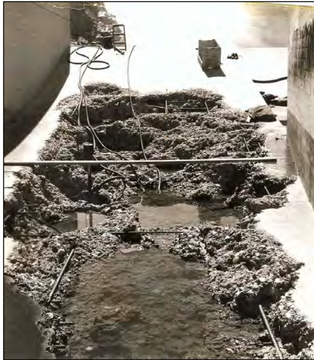
Figure A-47. —Discharge from the upstream slide gate resulted in significant cavitation damage to the invert of the flip bucket.
