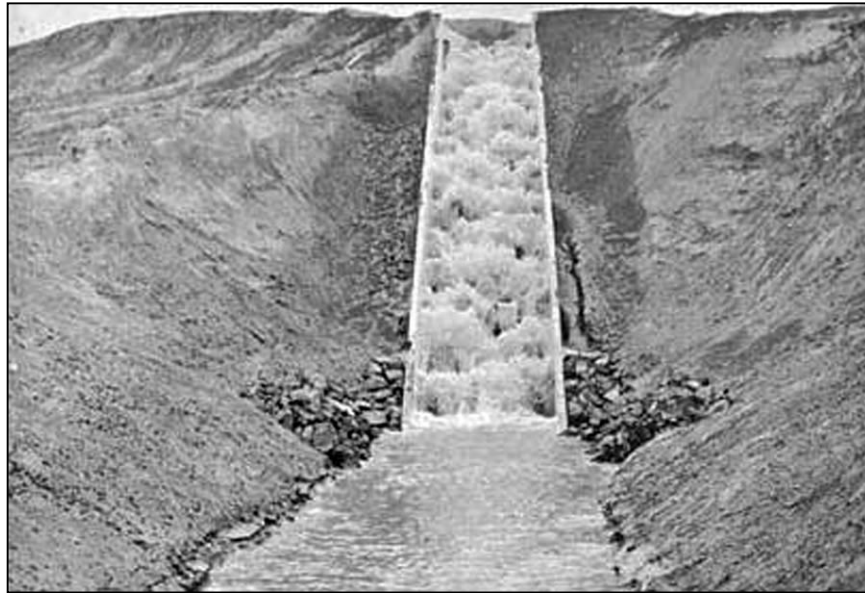
Figure 139. —This baffled drop has a chute that is 9 feet wide and 90 feet in length founded upon a 2:1 slope. The training walls are 5 feet high. The baffles are 18 inches high and wide with 18-inch spaces between them. The rows of baffles are all 6 feet apart ( Reclamation, 1984, p. 187 ).
