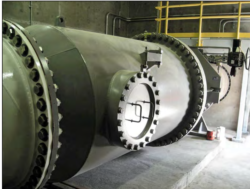
Figure 88. —The 48-inch diameter sleeve valve is located within a valve house and discharges directly into a horizontal stilling well. Photo courtesy of URS Corporation.
