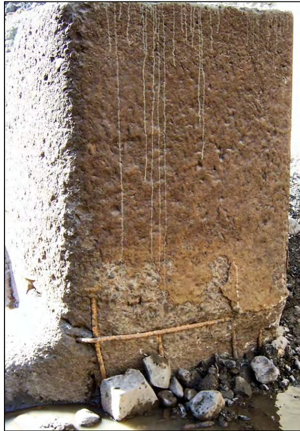
Figure 151.—The protective concrete cover has been removed exposing the reinforcement.
