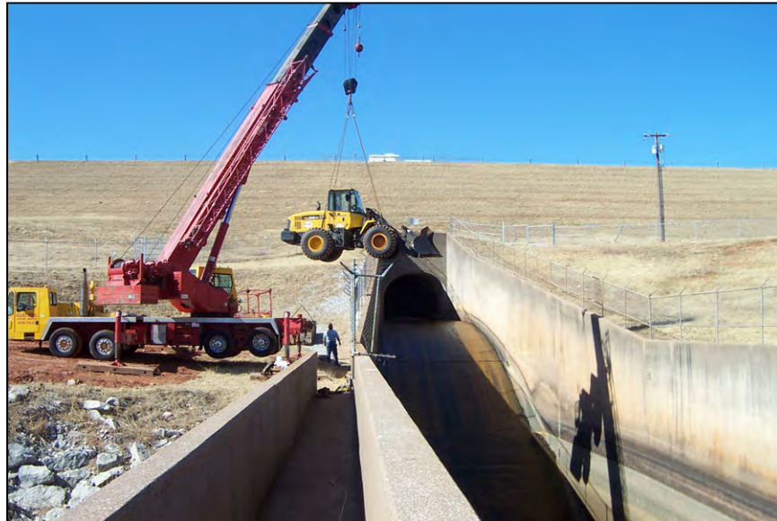
Figure A-62.—A crane was used to lower a front-end loader into the basin. The front-end loader was used to load debris into a metal container for removal.
