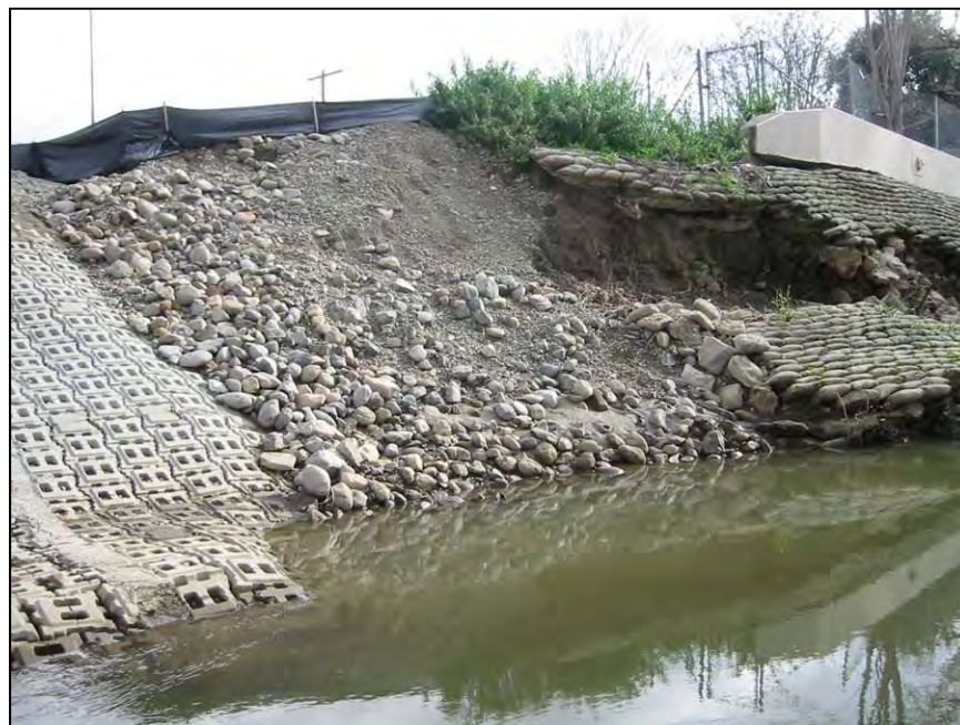
Figure A-30.—Eroded upstream bank.
