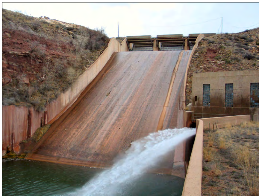
Figure 3.—An outlet works discharging into a spillway stilling basin.
