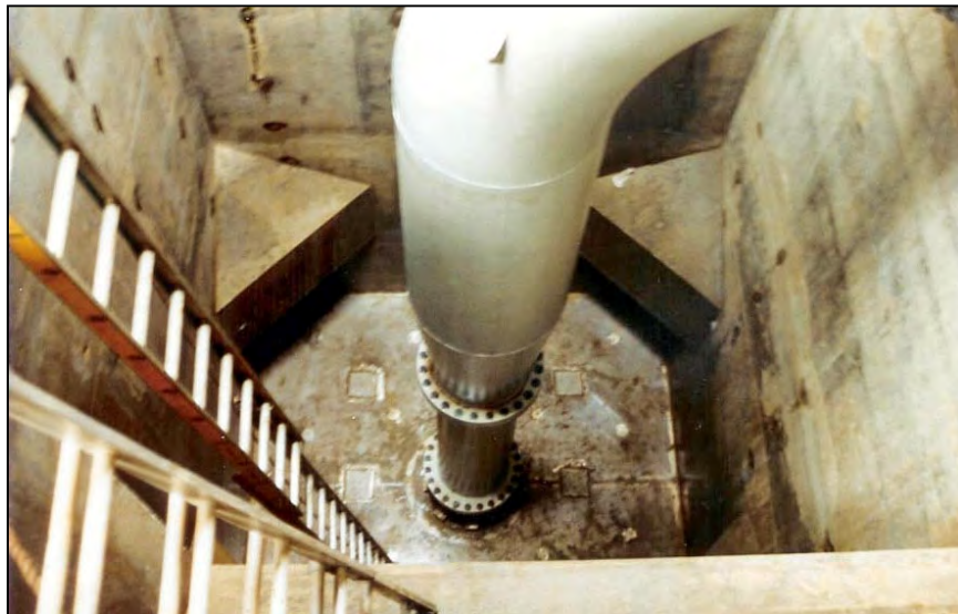
Figure A-74.—Stilling well at Palm Tree Creek Dam.
