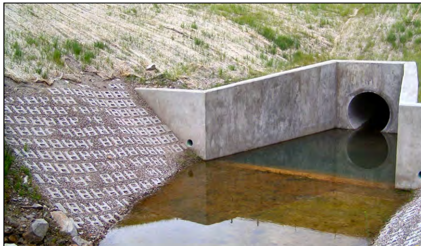
Figure 128. —Modified type PWD basin used with 48-inch diameter conduit with 45 feet of head. The discharge is operationally limited to 150 ft 3 /s.
