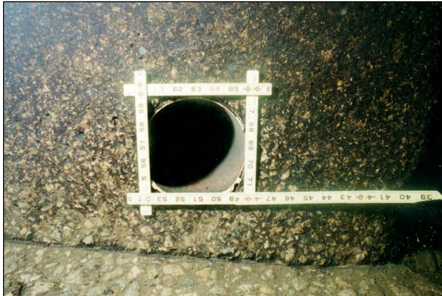
Figure A-107.—Typical condition of drain outfall in downstream face of outlet works stilling basin chute block. Note minor damage to exposed edge of PVC drainpipe likely due to movement of material in basin during releases.
