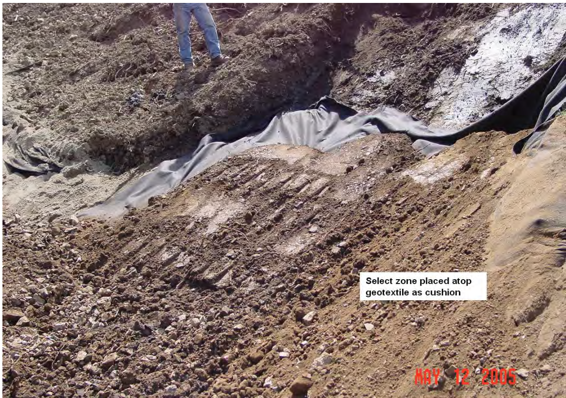
Figure 7 – C 33 sand placed below geotextile as filter and drain. The geotextile was covered with a cushion a fine grained soils with minimal angular coarse gravel particles to protect the geotextile from cuts and abrasion.
