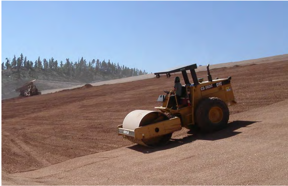
Figure 6.4.—Photograph showing compaction equipment preparing a suitably smooth and firm subgrade surface for geotextile placement.
