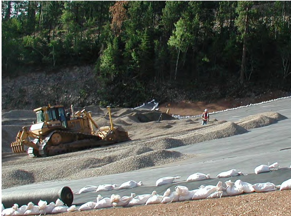
Figure 6.11.—Photograph of a low-ground-pressure bulldozer grading cover material to a uniform thickness of 1.5 feet. Note the presence of an inspector who is closely monitoring the covering operation.
