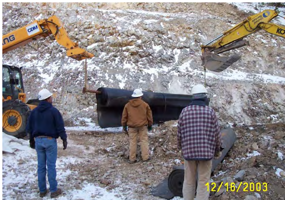
Figure 6.7.—Photograph of a steel pipe and slings being used to move a geosynthetic roll across a construction site to the installation area.
