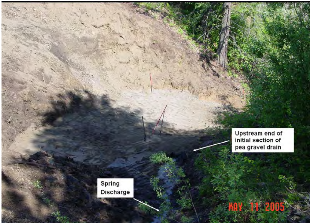
Figure 2 – The downstream segment of the geotextile wrapped drain has been placed and buried under a protective cushion of ASTM C 33 fine aggregate for concrete. The seep discharge from the abutment is still visible.
