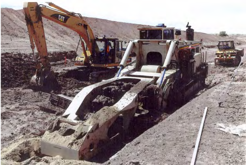
Figure MF3. Photograph of a trenching machine excavating a trench and backfilling it with a geotextile-wrapped pipe surrounded by a sand backfill.
