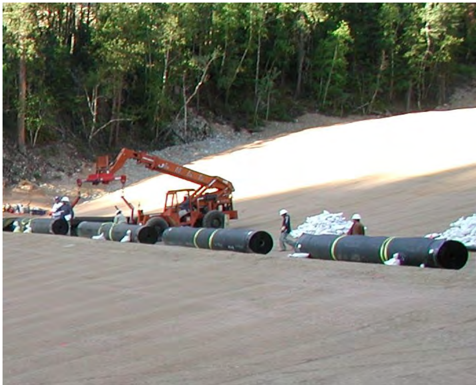
Figure 6.8.—Photograph showing preparations for geosynthetic installation. A swale is used to divide a long slope and provide an intermediate anchor trench location. Note the presence of proper equipment, sufficient labor, and adequate amounts of sand bags so materials can be efficiently installed and secured.
