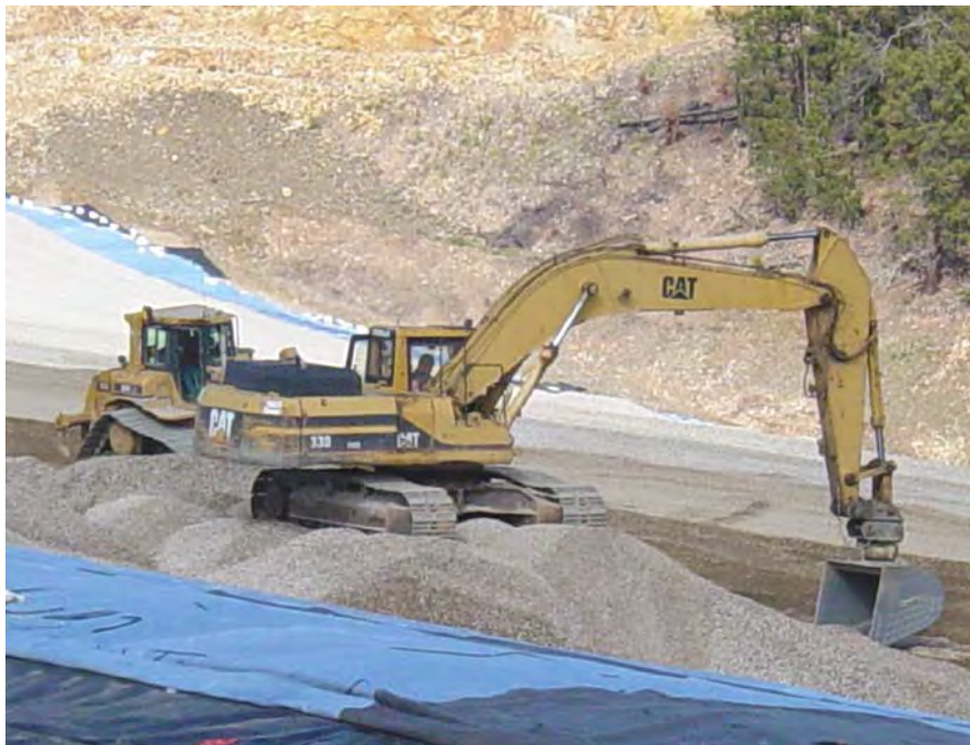
Figure 6.10.—Photograph of an excavator removing the tops of thick piles of cover material. Attempting to move such thick piles with a bulldozer is likely to damage the geotextile because of the high traction forces that would be required to push such a thick layer of material.
