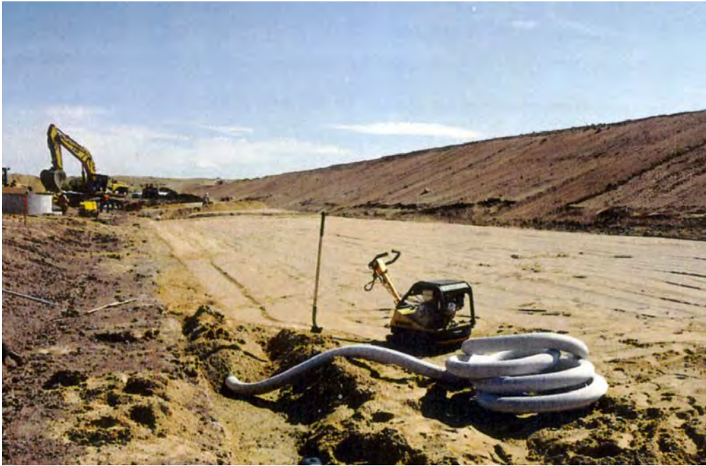
Figure MF5. Photograph of a geotextile-wrapped pipe emerging from a completed segment of the Many Farms dam toe drain trench.
