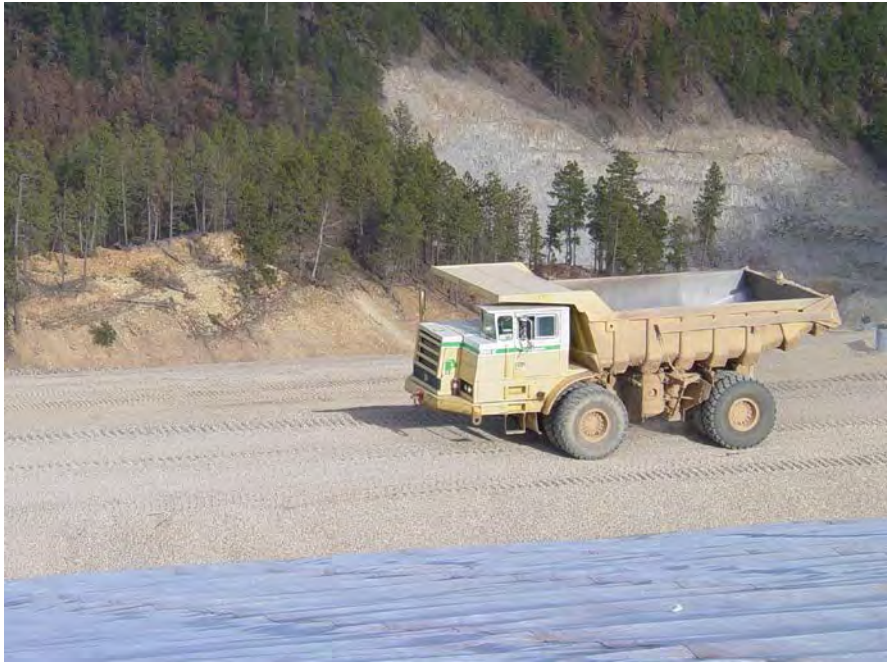
Figure 6.9.—Photograph showing a haul road where the cover layer has been temporarily increased to 5 feet to protect the geotextile from heavy equipment loading.
