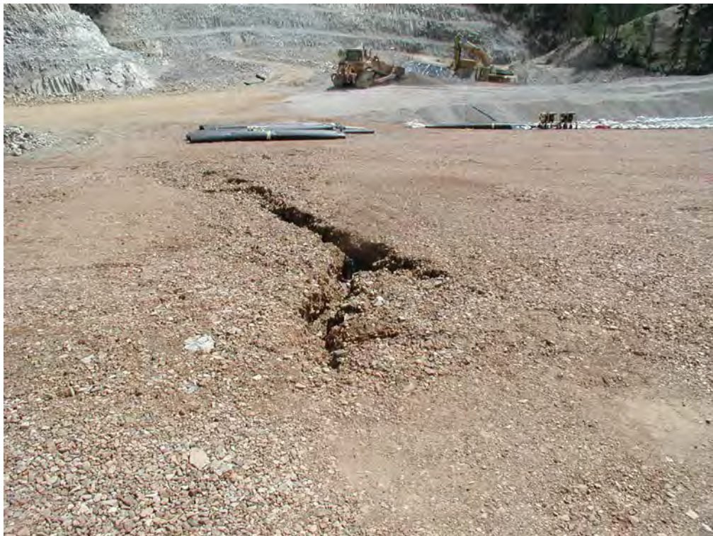
Figure 6.5.—Photograph showing a defect in a prepared subgrade surface. This portion of the subgrade was rejected by the inspector and had to be filled and smoothed.
