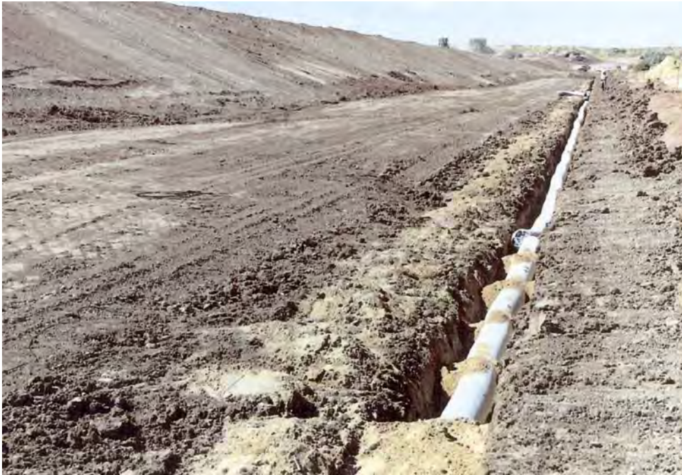
Figure MF4. Photograph of the toe drain trench showing geotextile-wrapped pipe without sand backfill. The trenching machine was so efficient that sand deliveries to the site could not keep up with pipe installation rates.
