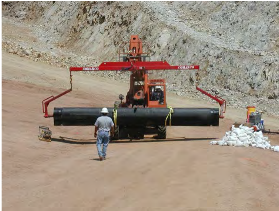
Figure 6.6.—Photograph showing moving a geosynthetic roll with a pipe and spreader bar, and a spotter. The spotter (person walking in front of the equipment) is needed to insure that the geosynthetic product does not strike any other objects which could damage the material.
