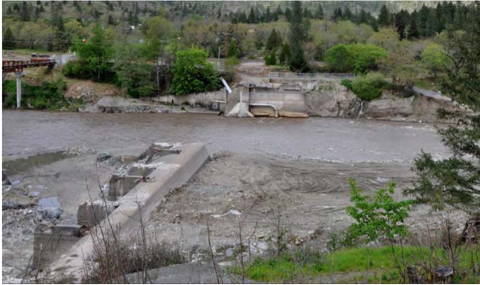
Figure 20.—A portion of Savage Rapids Dam (near Grants Pass, OR) was removed to allow fish passage while the remaining portion helps to protect a downstream pumping plant.
