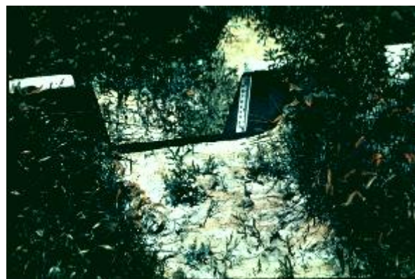
Figure 5-7 -- Sediment deposits in weir pool.
