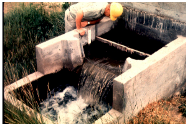
Figure 7-11 -- Weir box turnout with Cipolletti weir.
