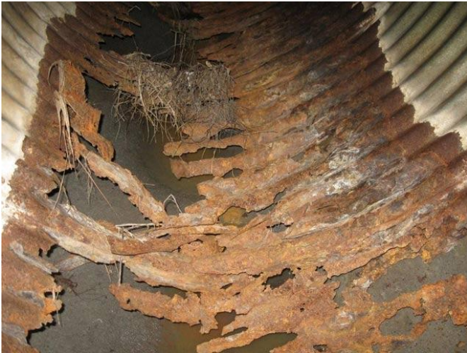
Photo 1: Severely deteriorated CMP. 1
