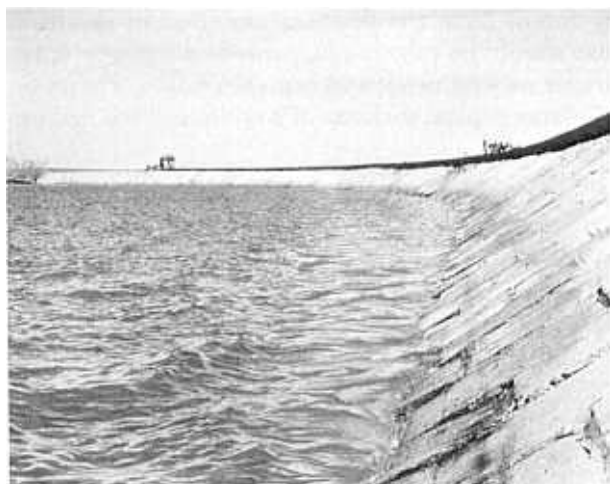
Figure 6.52.—Concrete paving blocks on the upstream slope of Belle Fourche Dam. Note the deteriorated condition of this paving after 40 years of service despite considerable maintenance. This dam is an earthfill structure on a tributary of the Belle Fourche River in South Dakota. 288-D-2937.
