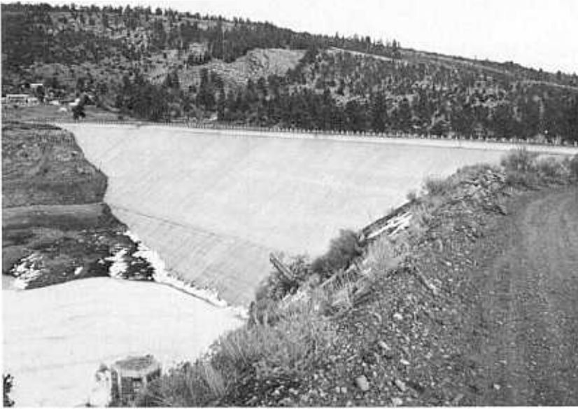
Figure 7-20.—Steel facing on the upstream slope of El Vado Dam, New Mexico. The facing is in excellent condition after 45 years of service. 288-D-2886.
