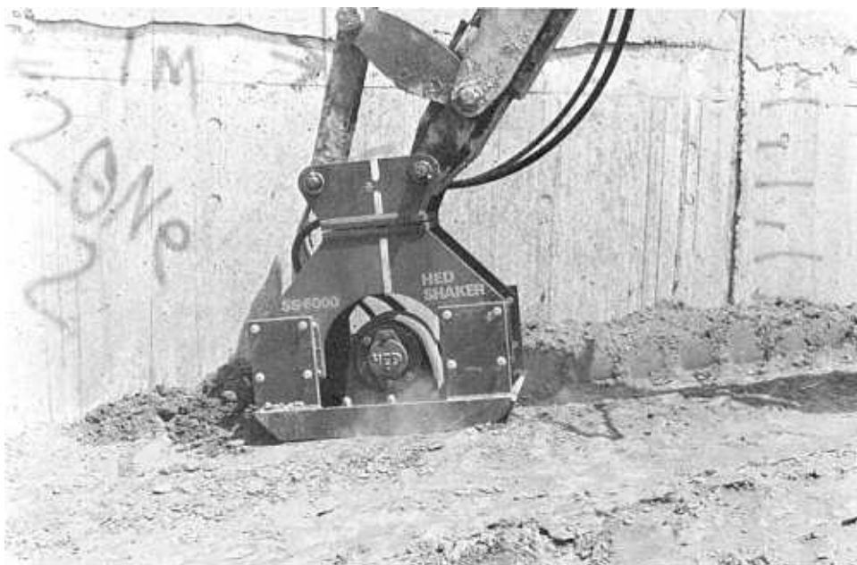
Figure E-6.—Vibratory plate being used for special compaction adjacent to conduit. McGee Creek Dam, Oklahoma. P801-D-81039.
