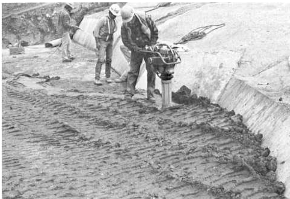
Figure E-4.—Use of formed dental concrete to fillet steep, rough rock. Special compaction against the steep surface. Ridgway Dam, Dallas Creek Project, Colorado. P801-D-81036
