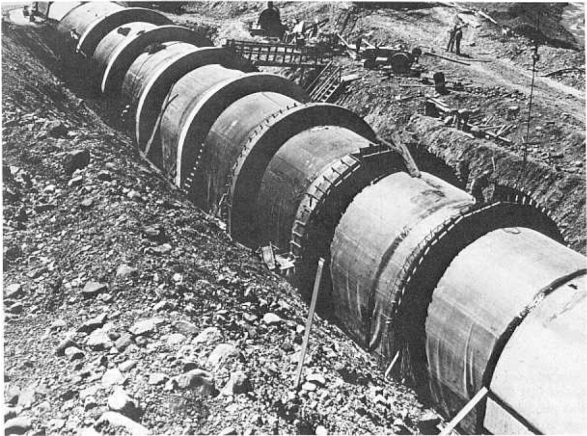
Figure 10-23.—Typical cutoff collars on an outlet works conduit. Silver Jack Dam, Colorado. P860-427-964NA.
