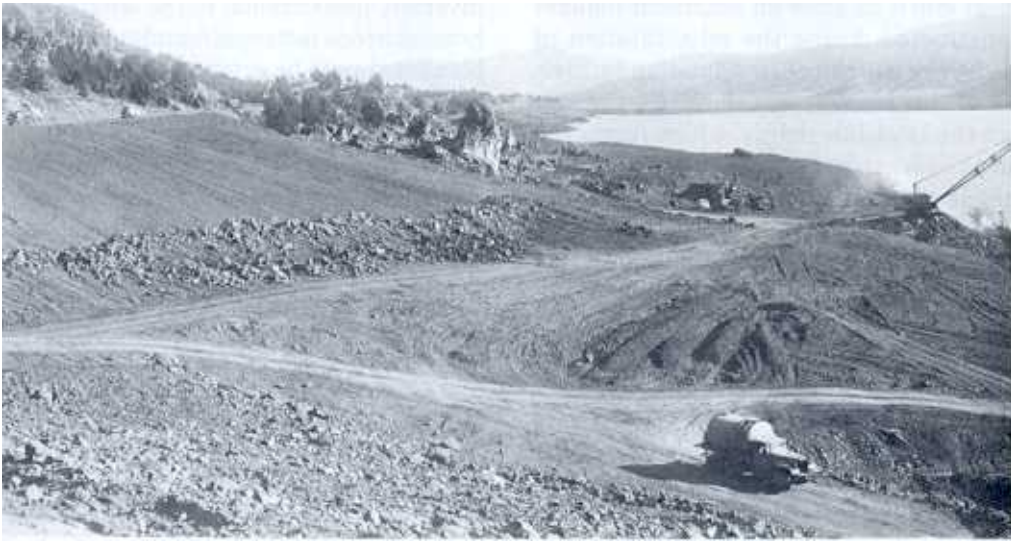
Figure 6-21.—Right abutment blanket construction at Ochoco Dam. On a tributary of the Crooked River in Oregon.
