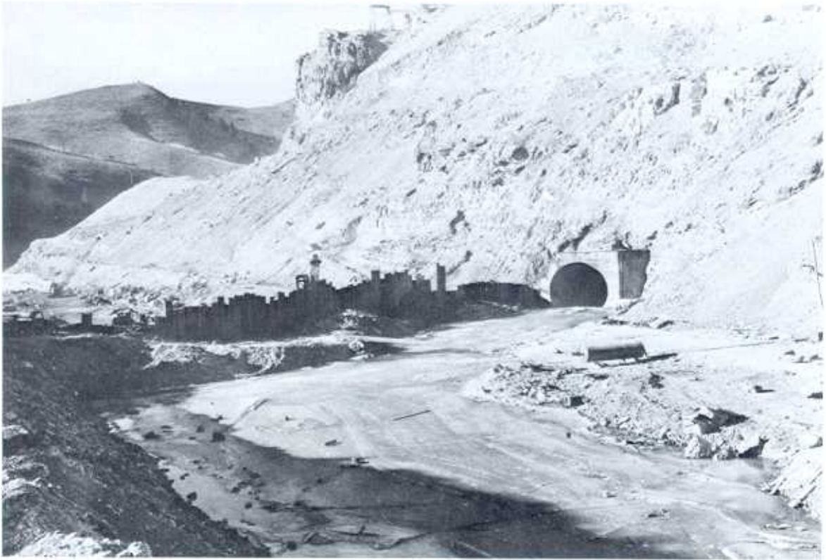
Figure 11-11.—Upstream cofferdam of steel sheet piling and earthfill diverting streamflow into tunnel. Green Mountain Dam. GM-283-CBT.
