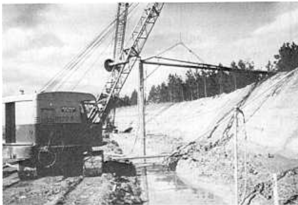
Figure 6-20.—Airlifting sand from bottom of slurry trench (U.S. Army Corps of Engineers). 288-D-2895.
