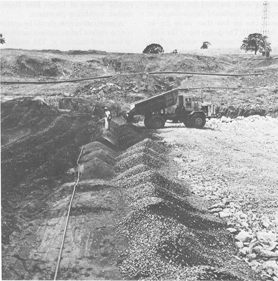
Figure 7-13.—Placement of fine and coarse filter material. For the 55-foot-high New Exchequer Saddle Dike, California. (Tudor Engineering Co. photograph). 288-D-2881.
