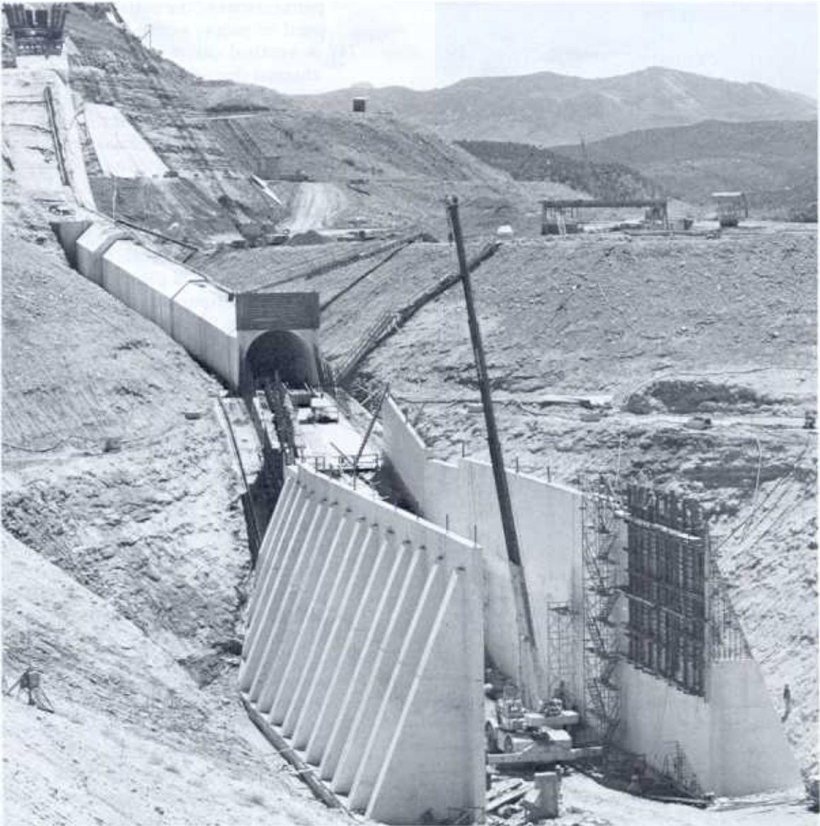
Figure 9-16.—Conduit and stilling basin for drop inlet spillway. Ridgway Dam during construction (1984). Dam is on the Uncompahgre River, Dallas Creek Project, Colorado. P894-427-6200NA.
