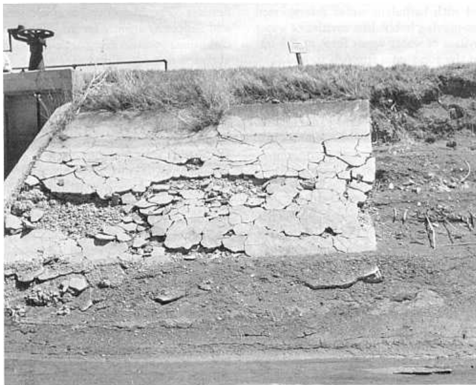
Figure F-2.—Disintegration of concrete caused by sulfate attack. PX-D-32050.
