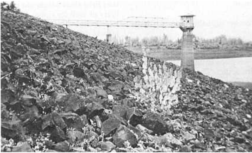
Figure 6-46.—Riprap on upstream slope of an earthfill dam. Dam is in excellent condition after 50 years of service. The structure is Cold Springs Dam, which forms an offstream reservoir on the Umatilla Project in Oregon. IO-2194.
