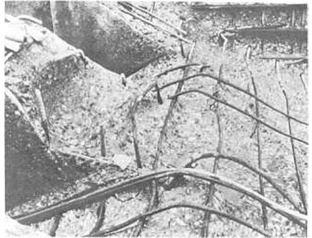
Figure F-4.—Abrasion erosion of concrete in the dentates, walls, and floor of the Yellowtail Afterbay Dam sluiceway stilling basin. The "ball-mill" action of cobbles, gravel, and sand in turbulent water abraded the concrete, thus destroying the integrity of the structure. P459-D-68905.
