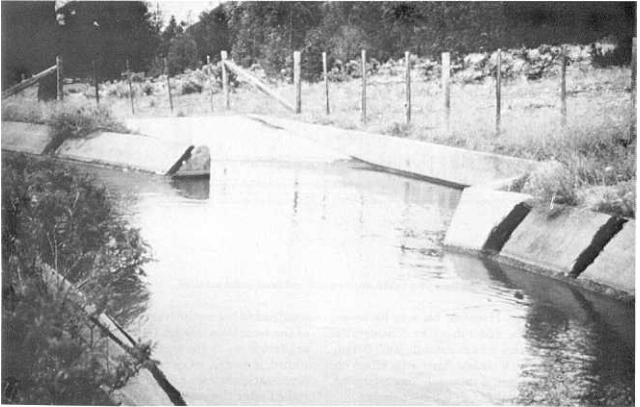
Figure 2-12. Revised Richmond deer-escape ramp. Water flow is from left to right. From [14]. P801-D-81031
