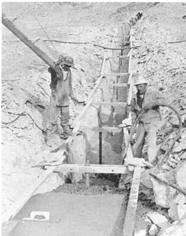
Figure 6-12.—Placing concrete grout cap at Navajo Dam, New Mexico. The 2-inch-diameter grout nipples are fixed at 10-foot intervals. 711-422-250.
