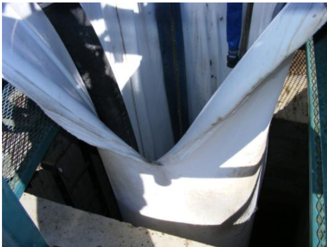
Figure 5 – CIPP installed through gate tower (White pipe is the CIPP and black pipe is used to circulate hot water for curing)
