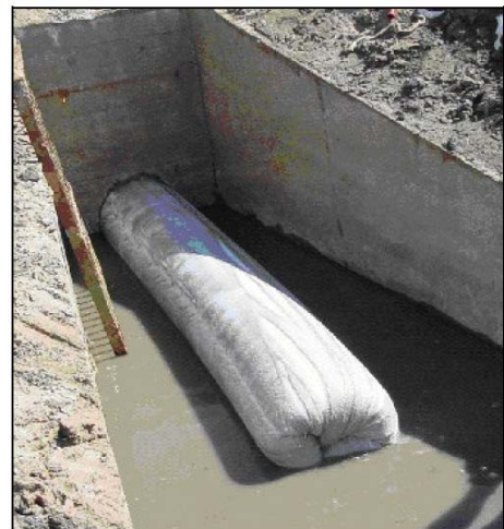
Figure 3. CIPP liner exiting from an existing conduit via the hydrostatic inversion method [5]
